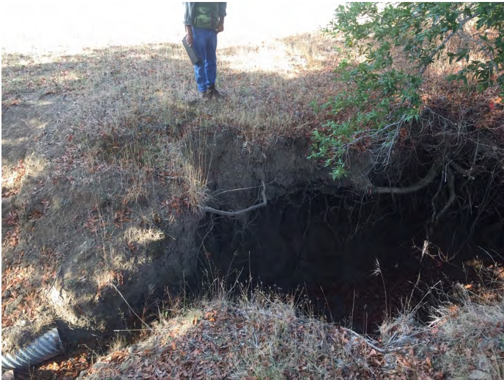
Figure 7. Approximately 10 feet of channel incision at culvert outlet along west-side tributary. Photo taken just upstream from Figure 8.
