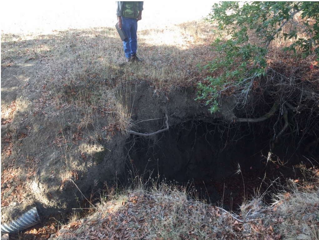
Figure 7. Approximately 10 feet of channel incision at culvert outlet along west-side tributary. Photo taken just upstream from Figure 8.
