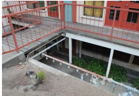
Figure 20: Garden level below a pedestrian bridge accessing the mezzanine level of Building 1.
