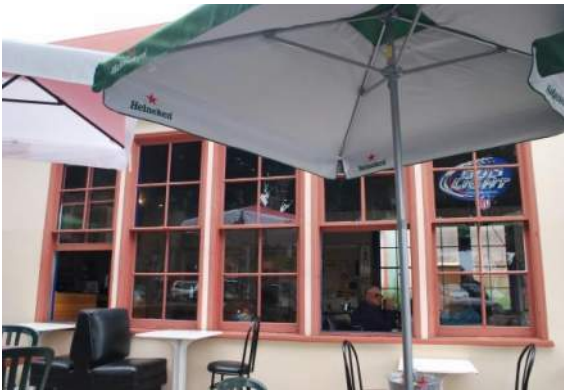
Figure 6: Bank of five single-hung multi-lite wood windows on the southeast façade of Building 0.
