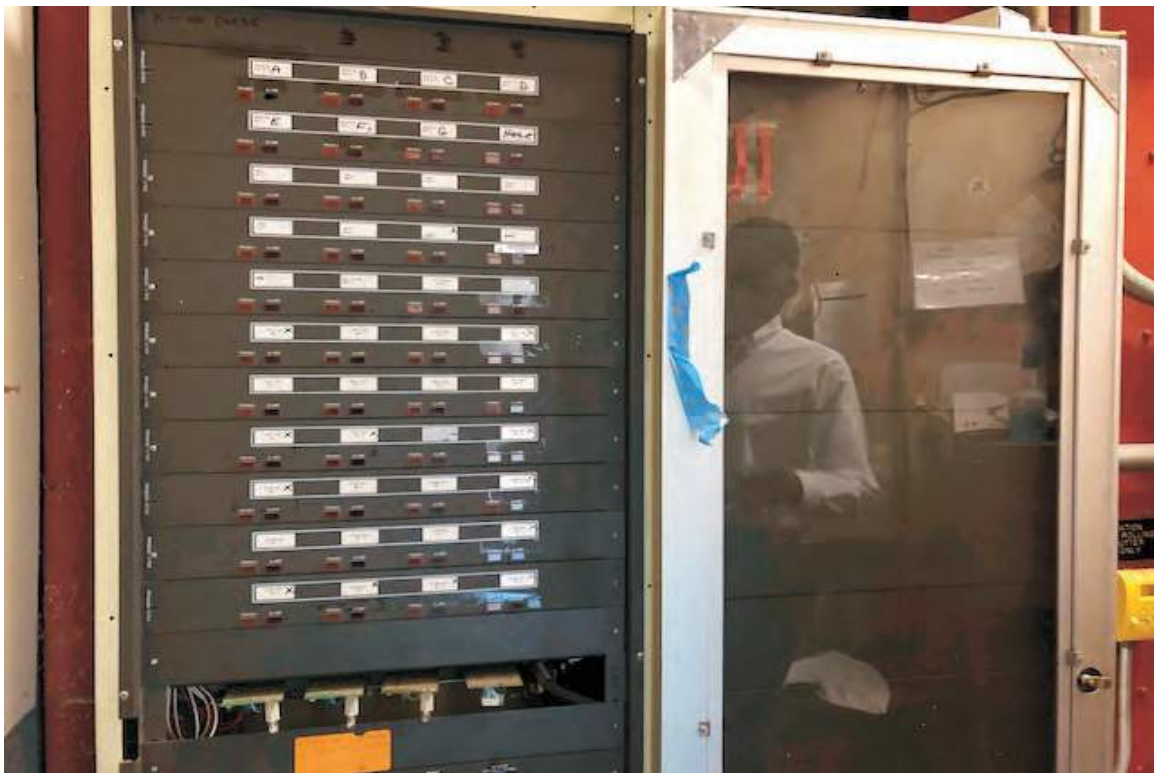
Photo 24: Fire safety monitoring equipment room.
