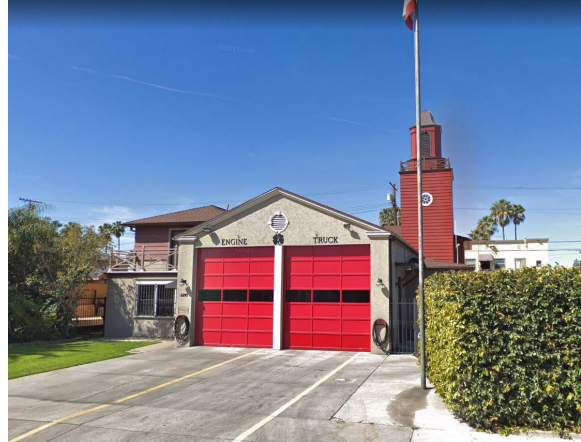
Figure 27: Station No. 7 has been altered with the removal of exterior siding, application of textured stucco and replacement windows, 2019 (Google Street View)
