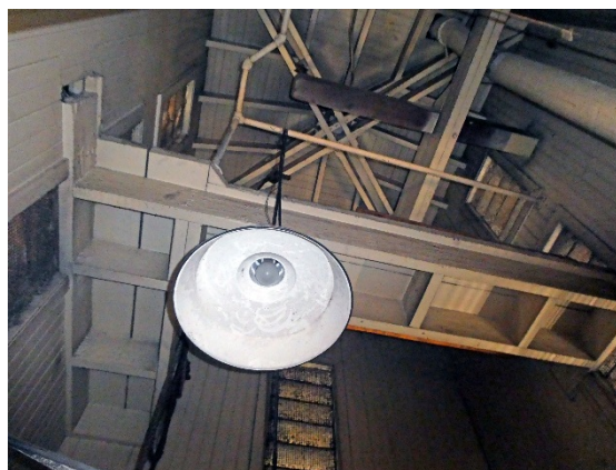
Figure 28: Top of hose tower, showing walking platform, metal pipe railing and hose rolling mechanism (GPA, 2019)
