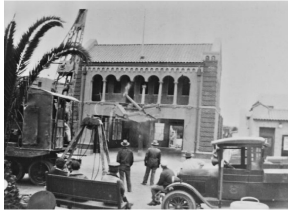
Figure 22: Station No. 9 was demolished along with all other unsafe structures, date unknown (CSUDH Archives)
