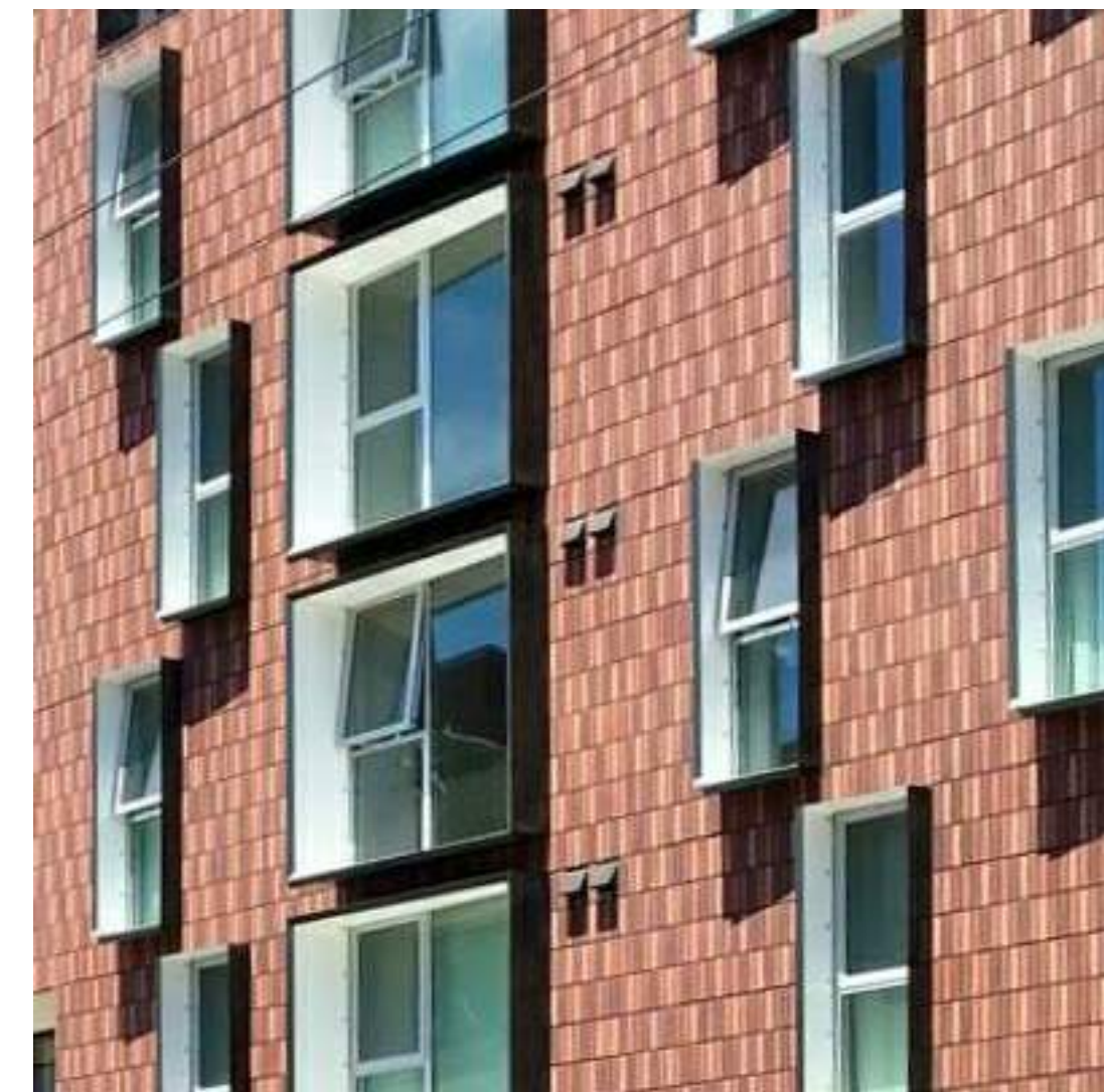
POWDER-COATED SUNSHADES DARK WARM EXTERIOR COLOR, LIGHT INTERIOR COLOR SELECT SOUTH AND WEST WINDOWS
