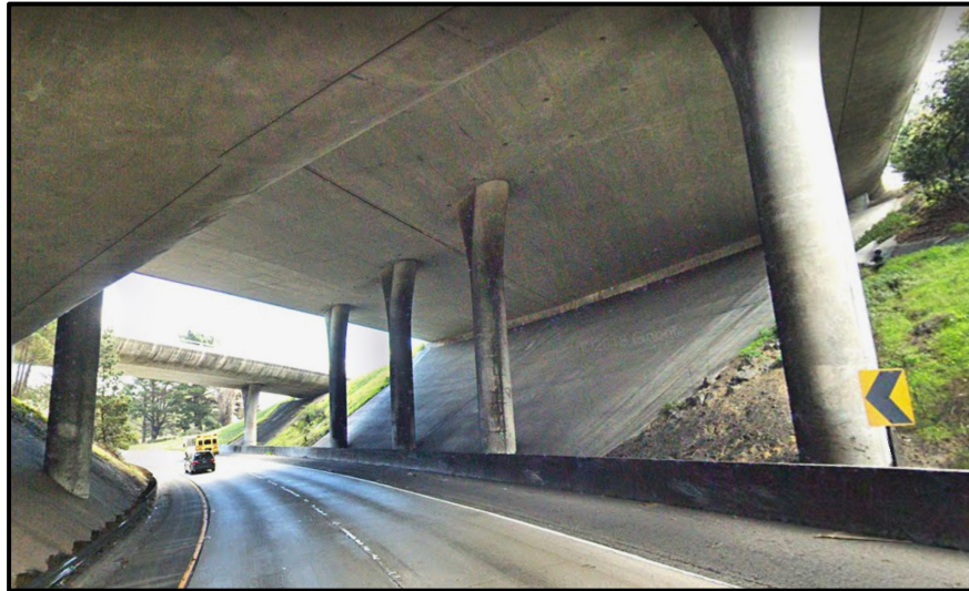
Photo 8: I-280/I-380 Separation Bridge; View from EB I-380 of Bent 3 and Bent 2 of the (I-280) Bridge. Slope paving is visible on the right side of the image behind the columns.
