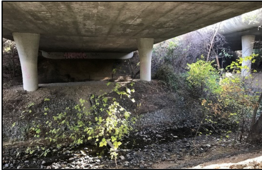
Photo 3: Alpine Road UC (L/R) Bridges; View south of Bent 2 and Los Trancos Creek
