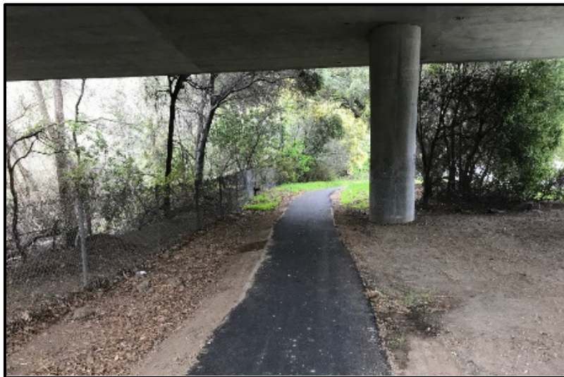
Photo 2: Alpine Road UC (L/R) Bridges; View WB of Alpine Trail and chain-link fence, and a column from Bent 3 (left bridge)
