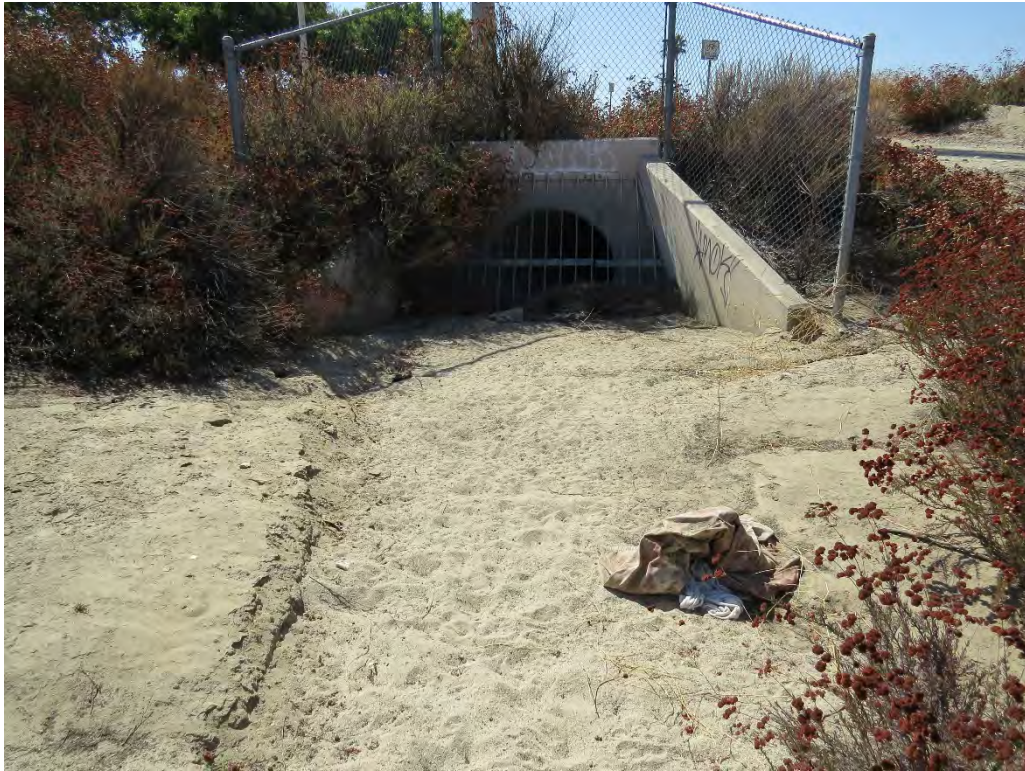
Photograph 11: View of the of the terminus of Drainage 1 at the culvert on the southwest corner of the site.
