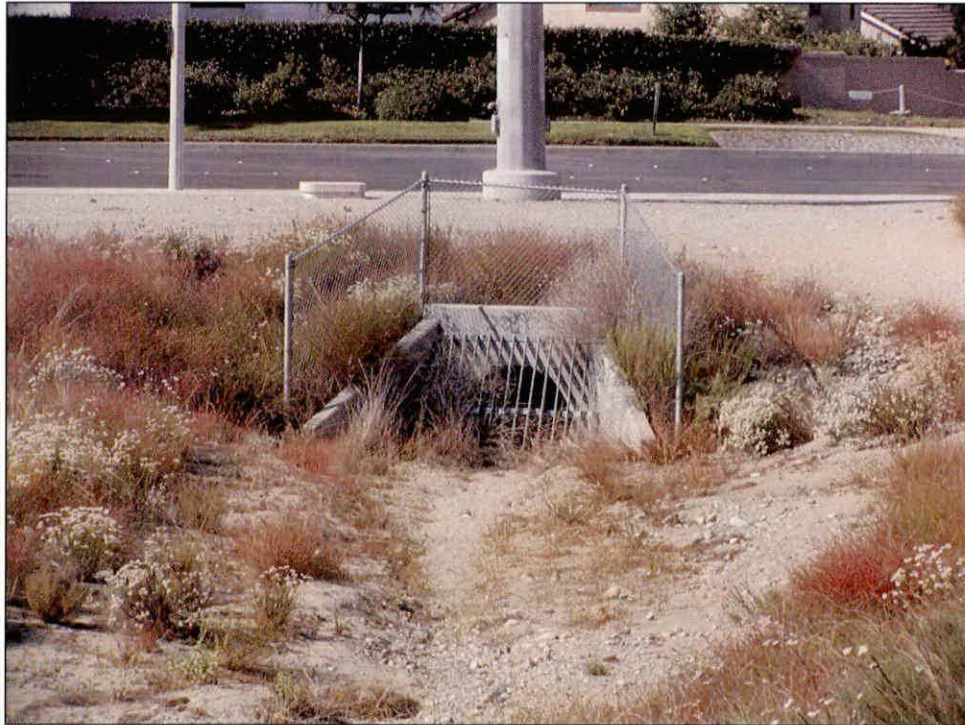
PHOTOGRAPH 7: View of drainage feature and culvert on project site as seen facing Base Line Road (south boundary).
