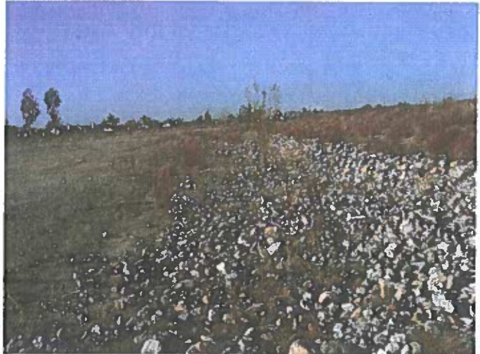
Photo 2: Channelized portion of Drainage A, lined with imported cobble and river-rock looking southwest.
