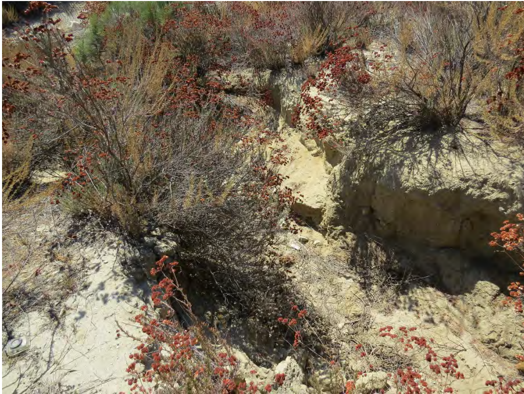
Photograph 19: View of Drainage 2 where it is more incised on the bank of Drainage 1.
