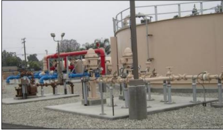
Figure 8-20: Water Treatment Facility, Rubidoux Community Services District
