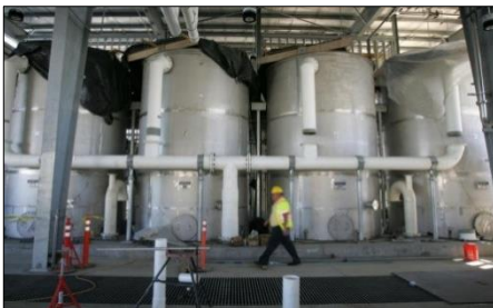
Figure 8-19: Water desalter plant, Jurupa Valley (Press-Enterprise)
