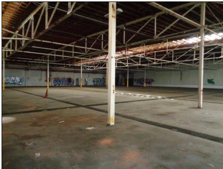
Figure 5-28. Star-Kist Plant No. 4, interior, warehouse/manufacturing area showing drains in floor, camera facing southeast.
