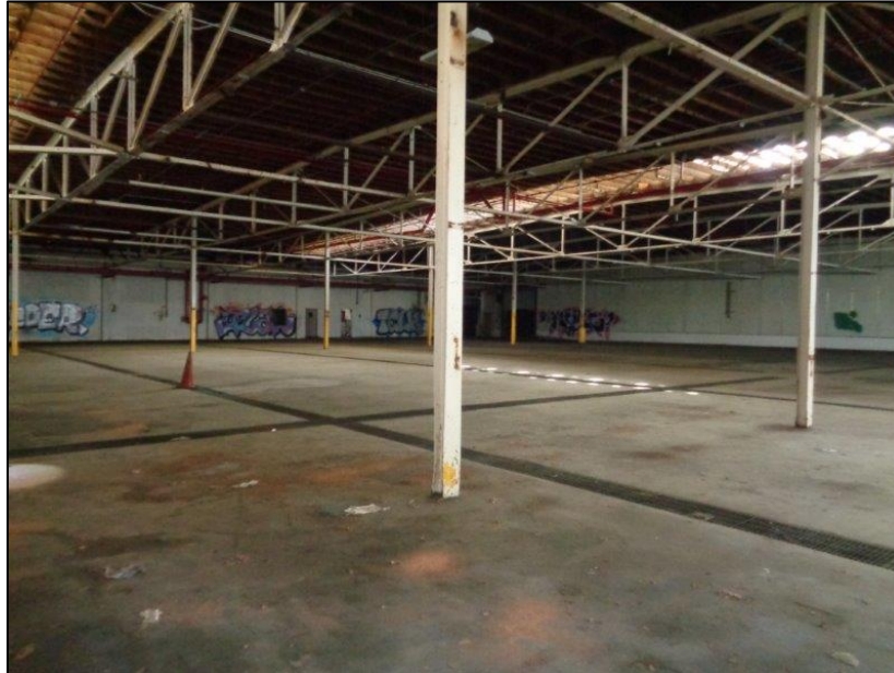
Figure 27: Star-Kist Plant No. 4, interior, warehouse/manufacturing area showing drains in floor, camera facing southeast. ICF, 2018.
