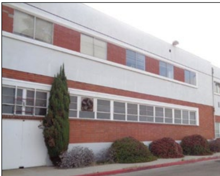
Figure 6: Star-Kist Plant No. 4, primary (west) elevation, detail of third building from the north, south wing, camera facing east. ICF, 2018.
