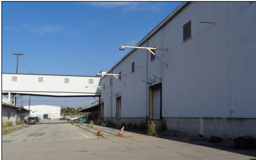
Photograph 2: West elevation, Can Manufacturing (formerly Impress) portion of facility in distance (left), sky-bridge to Star-Kist Plant No. 4 Main Facility and Empty Can (formerly Green Building) (center) and Warehouse (formerly Distribution) portion of facility in foreground (right), camera facing north. ICF, 2018.
