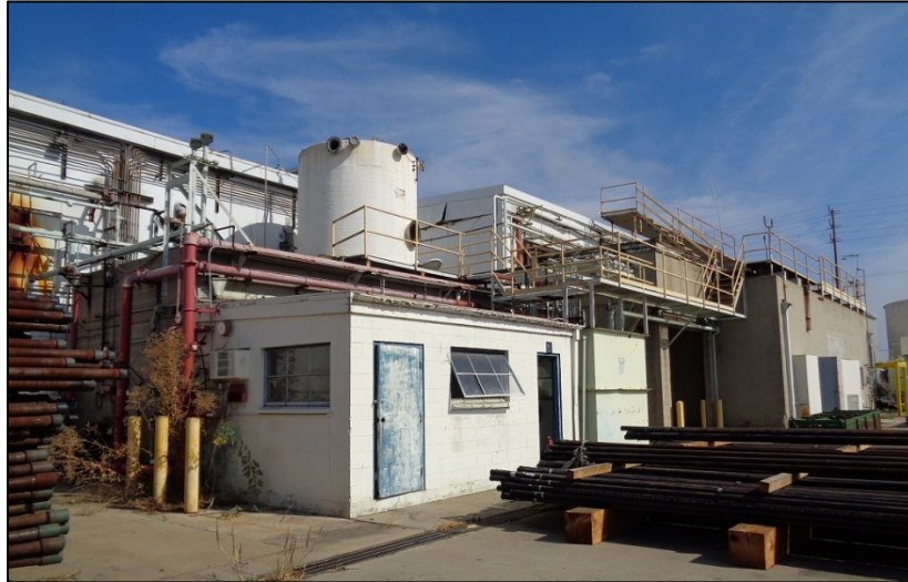
Photograph 5: South elevation, Cold Storage portion of the facility, camera facing northeast. ICF, 2018.
