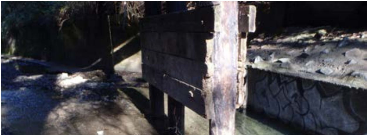
View 3. View of Meadow Way Bridge lower wood beam connecting structure to foundation.
