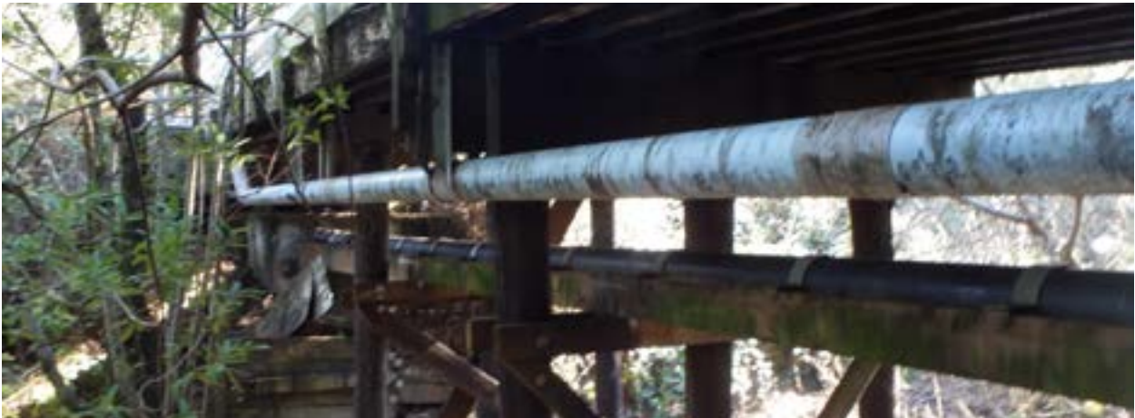
View 2. View of Meadow Way Bridge structure. The guard rail for the upper driving structure is visible in the photo.
