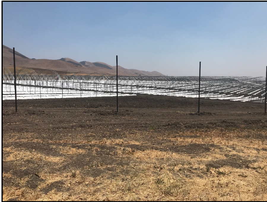
Photo 3. Hoop houses constructed on the eastern end of the project site (Site 1), view south (August 6, 2018).
