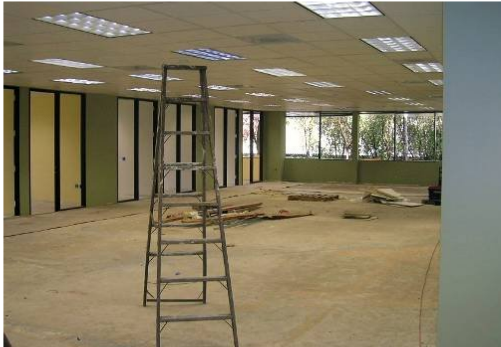
17 View of a major renovation undergoing in one of the buildings in the Subject.
