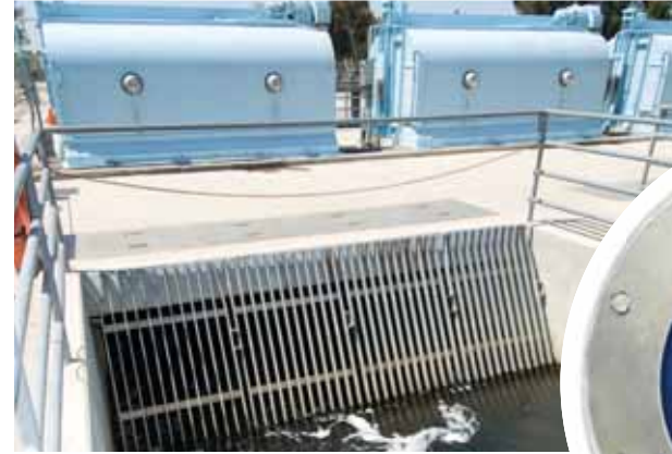
4 Screening Los Angeles Aqueduct Filtration Plant (LAAF) Inlet Structure Water flows through the inlet of the LAAF, where large pieces of debris or algae are removed by screens.
