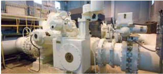
12 Local Pump Station Fletcher Pump Station Additional chlorine is added before large pumps send the water to L.A. neighborhoods, east of Ivanhoe Reservoir.
