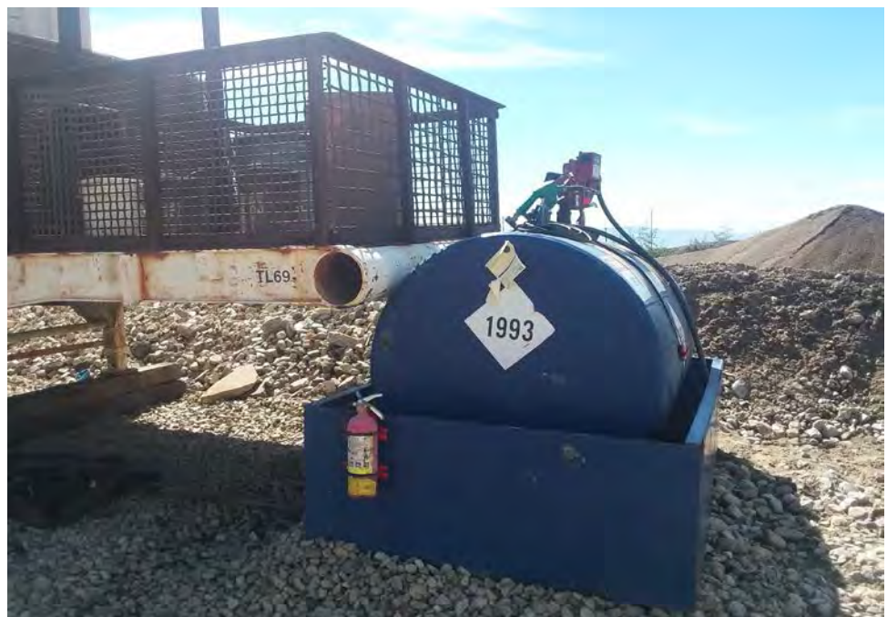
Photograph No. 4: On-site 500-gallon fuel aboveground storage tank in secondary confinement.
