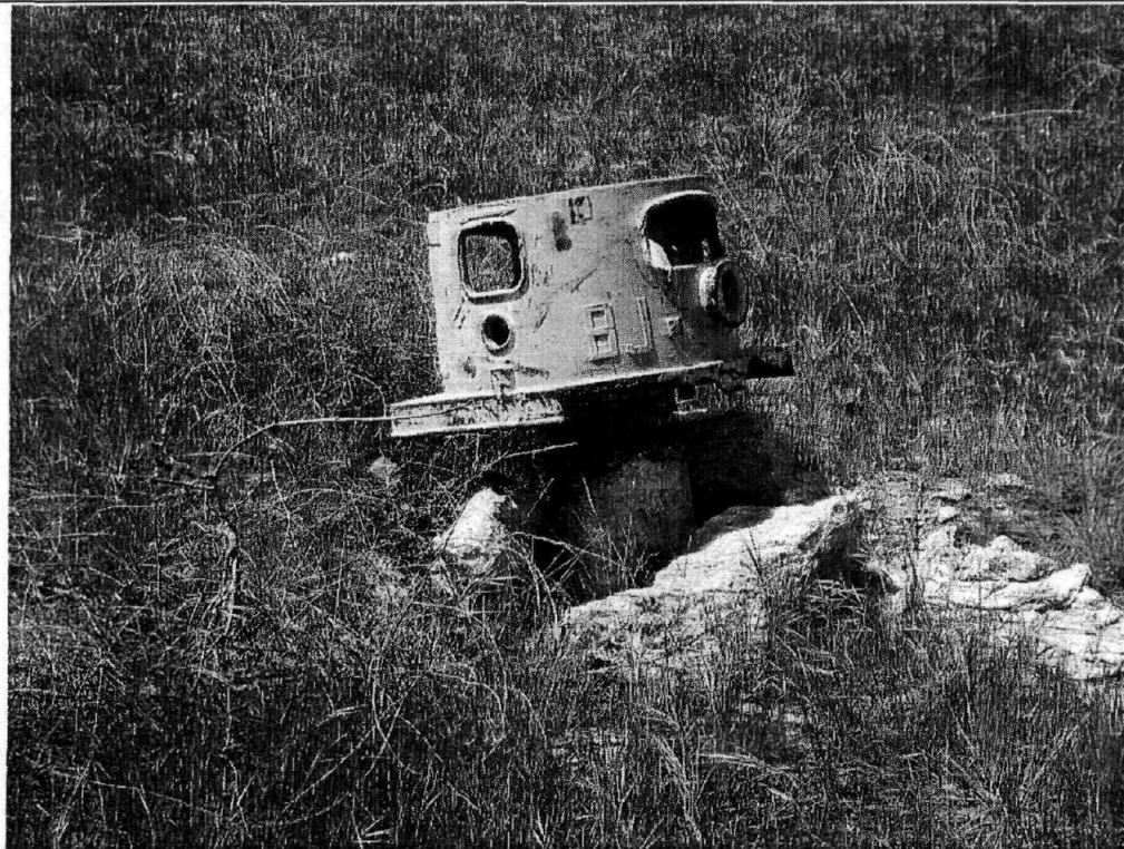
Large steel pipe junction. View toward west, 4/12/2006. Photo No. 3.
