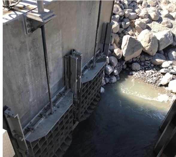
The Windy Point intake/slucing structure is used to manage sediment loads in the water before it reaches the 19 replenishment ponds.
