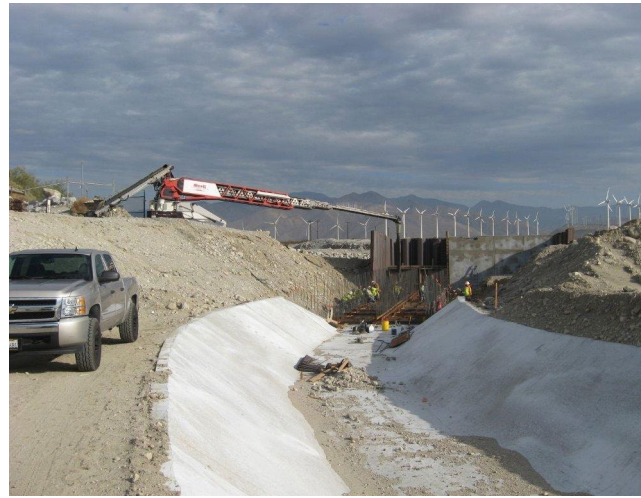
In 2013, CVWD completed construction of a new intake/slucing structure and a 12,000-foot-long concrete-lined conveyance channel as well as groundwater replenishment pond improvements.
