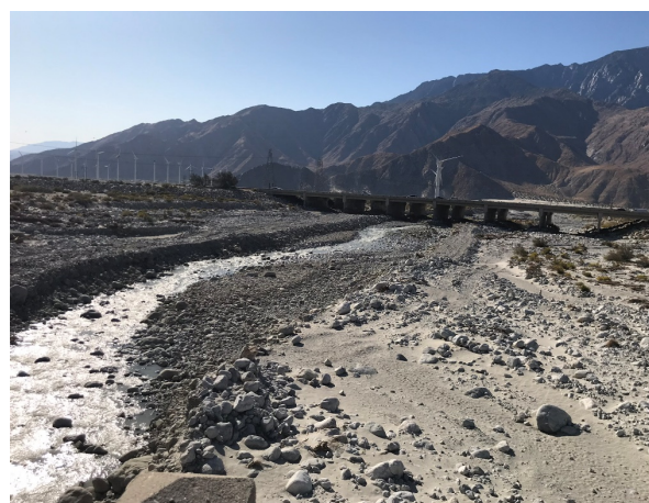
Colorado River water is conveyed along the 5-mile-long earthen channel, beneath I-10 to the Windy Point intake/slucing structure.
