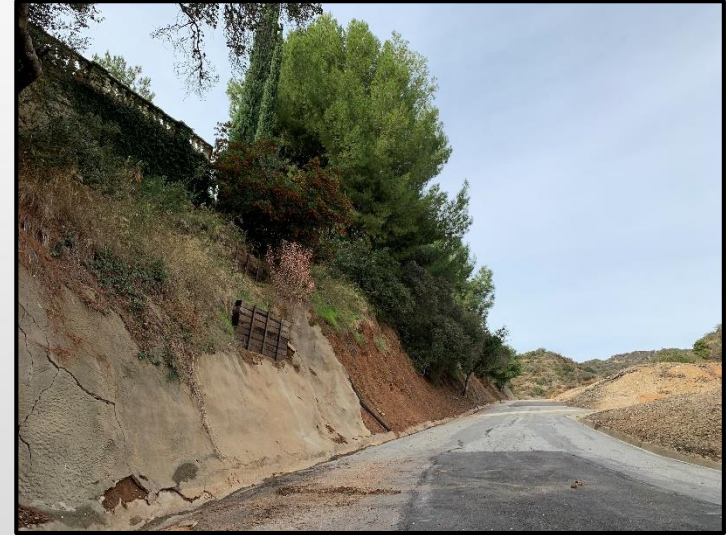
Photograph 16. Photograph of existing Flood Access Road adjacent to the Spinks Disposal Area, in the southwestern portion of the Project site. Photograph taken facing northwest.
