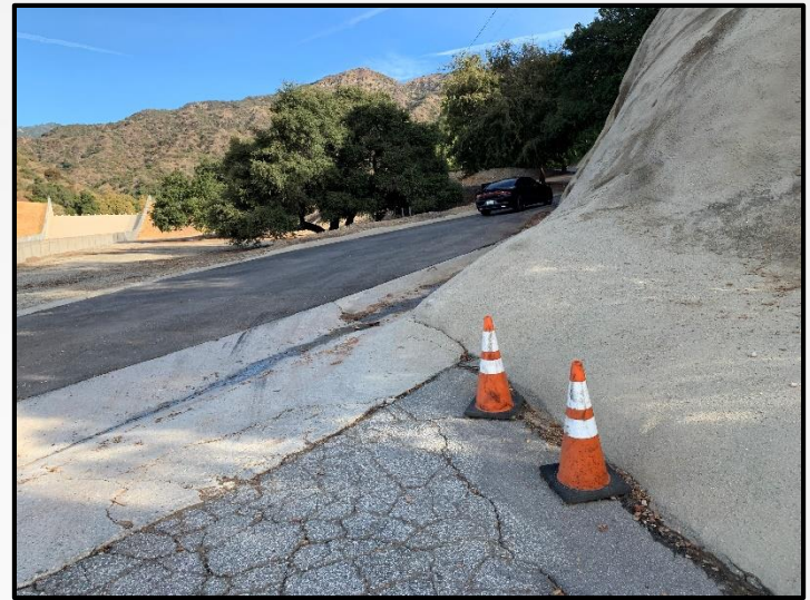
Photograph 2. View of existing Flood Control Road at the entrance of the Project site. Photograph taken facing north.
