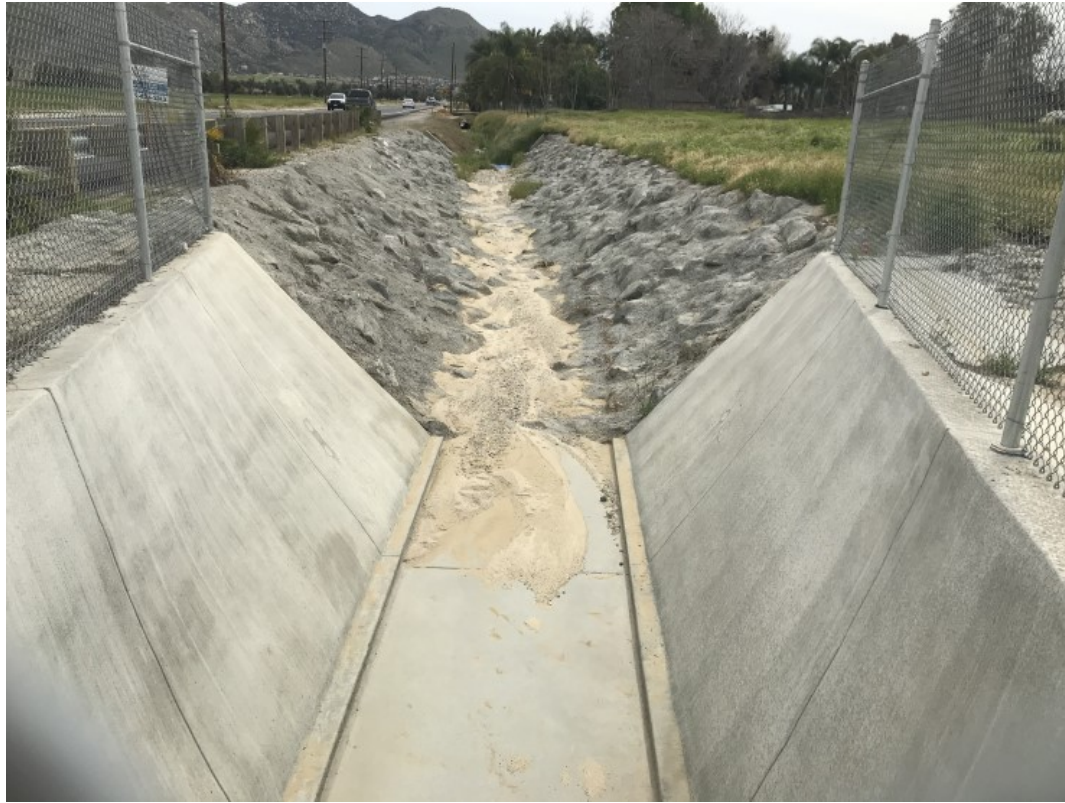
Photograph 9: 03-31-20. Start of improved portion of ephemeral storm drain ditch looking south.
