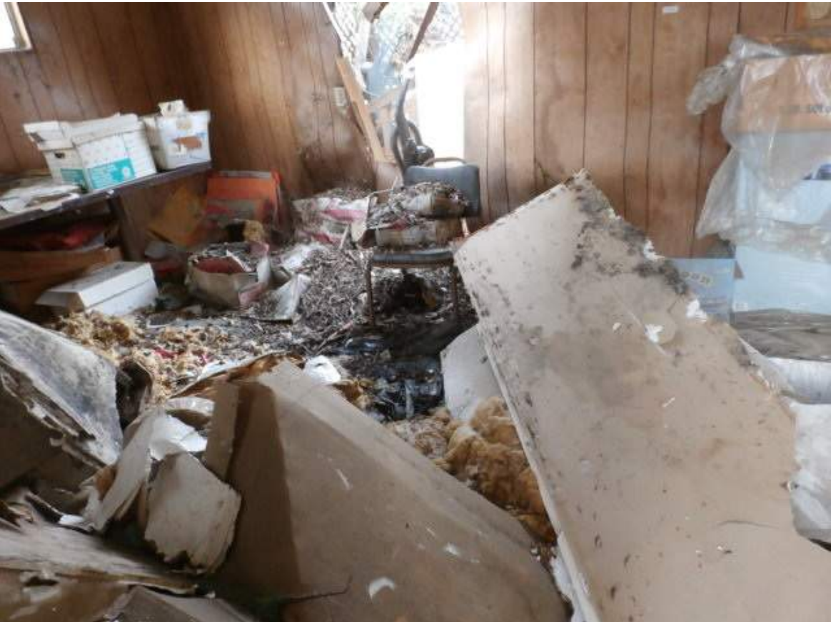
PHOTO 24 SHOWING THE INSIDE OF THE GARAGE ASSOCIATED WITH THE RESIDENCE ADDRESSED 12981 REDLANDS. PART OF THE GARAGE IS DAMAGED.
