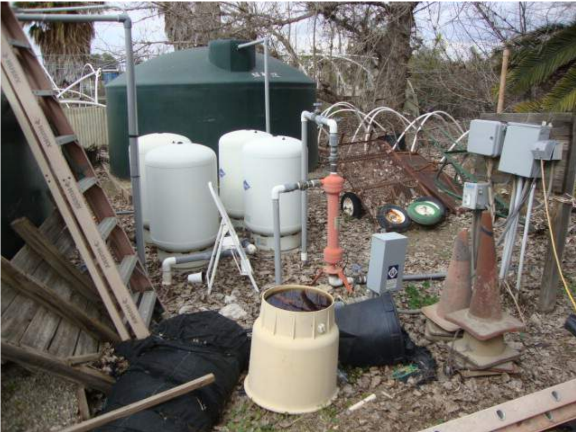
PHOTO 36 VIEW OF THE WATER WELL, BLADDER TANKS, HOLDING TANKS AND FILTERS. PUMP IS ELECTRIC.
