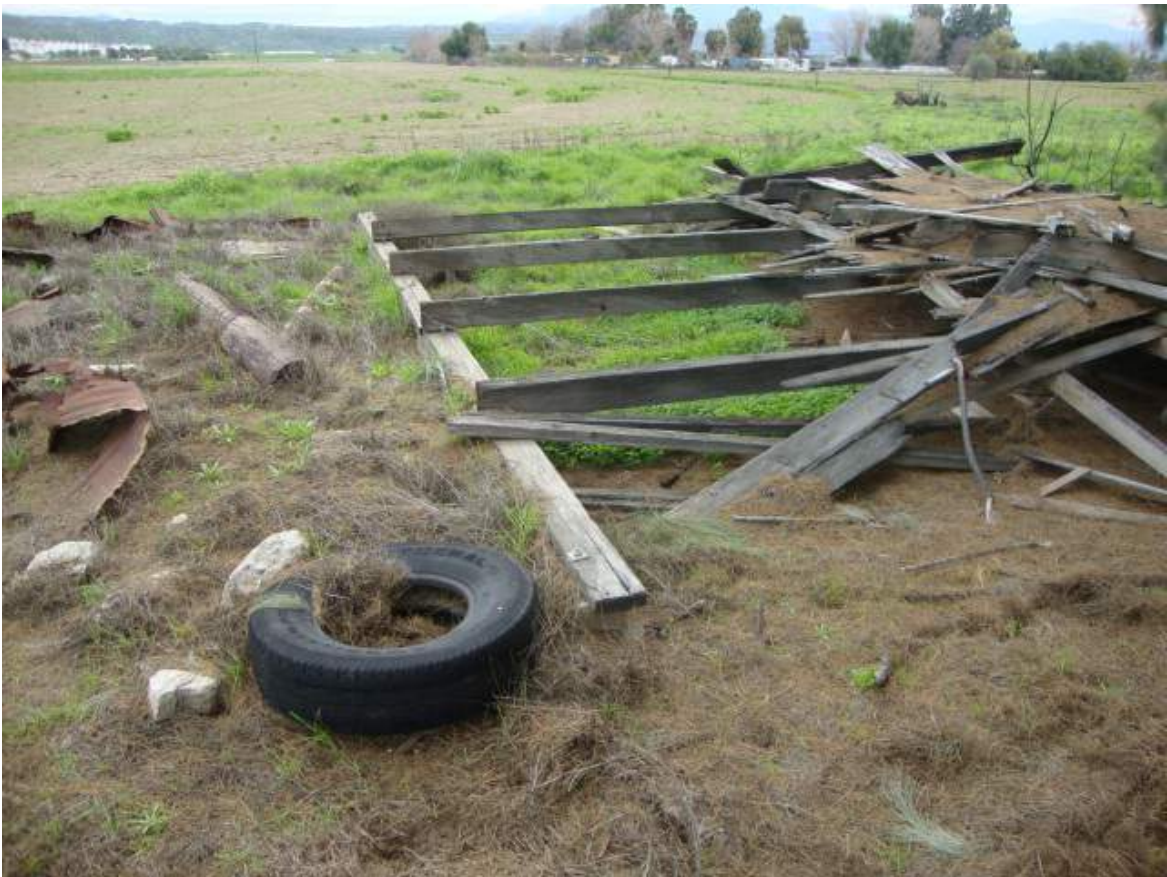
PHOTO 19 VIEW FACING EAST SHOWING THE WOODEN FOUNDATION NOTED IN THE PREVIOUS PHOTOGRAPH.
