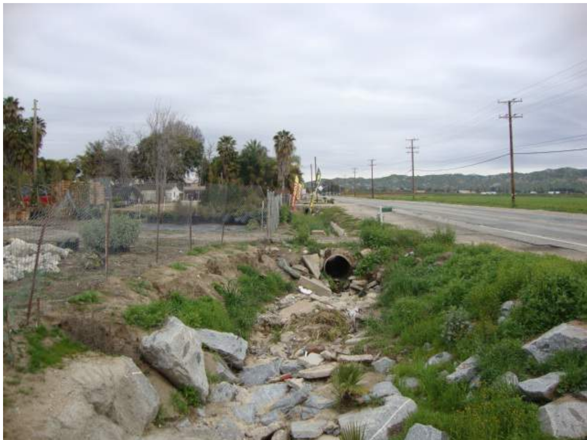
PHOTO 22 VIEW FACING NORTH FROM THE INTERSECTION OF ENCELIA AVE. AND REDLANDS BLVD. SHOWING HALLS NURSERY TO THE LEFT ( WEST) AND REDLANDS BLVD. TO THE RIGHT WITH THE EARTHEN CHANNEL ALONG THE ROADWAY.
