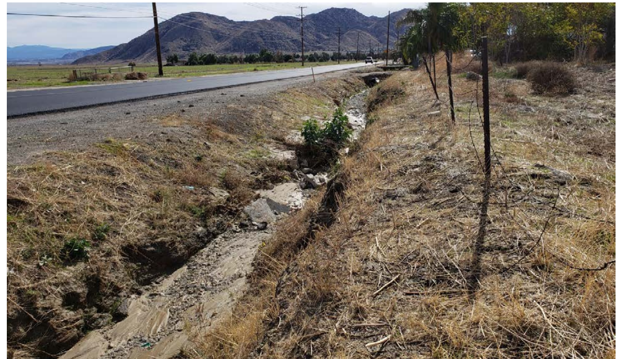
Photograph 4: Photo of Drainage Ditch 2 running parallel to Redlands Boulevard. Note the lack of vegetation.
