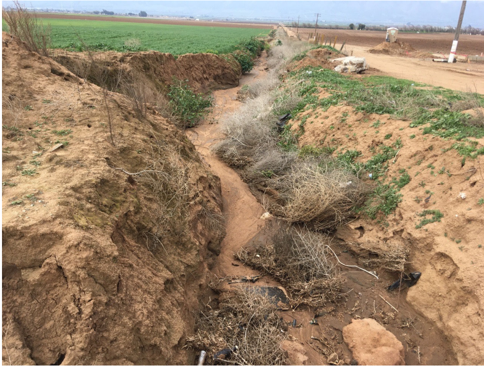
Upstream end of Ditch 1, which was claimed as a water of the U.S. in 2014. No flows were evident during the January and March 2021 site visits.
