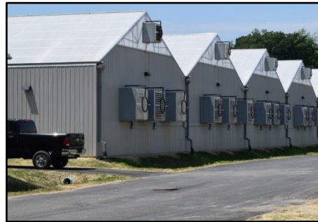
FogCo installed on greenhouse exhaust vents.
