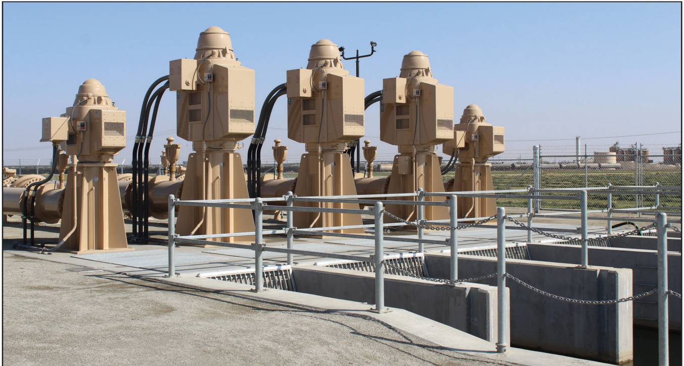
Typical Pump Station Facilities
