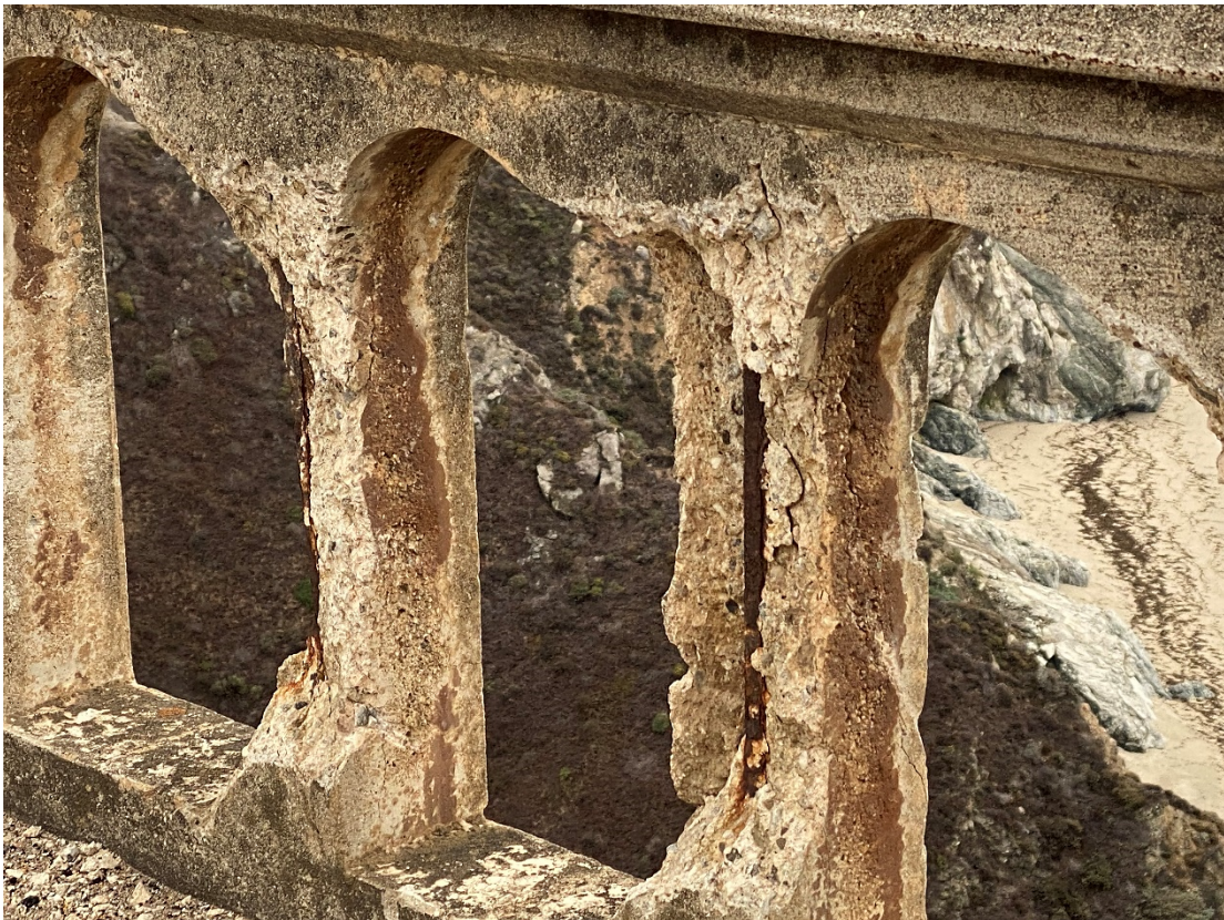
Figure 1-2 Photo of Bixby Creek Bridge Rail Deterioration
