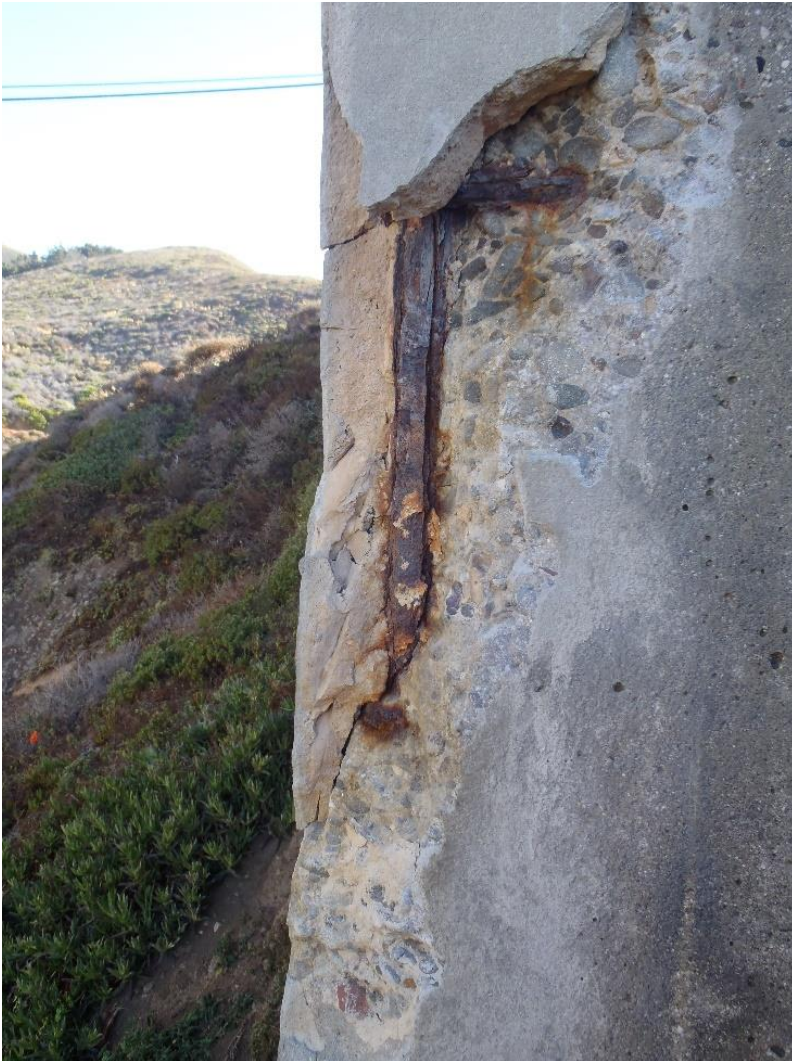
Figure 1-5 Photo of Garrapata Creek Bridge Rail Deterioration
