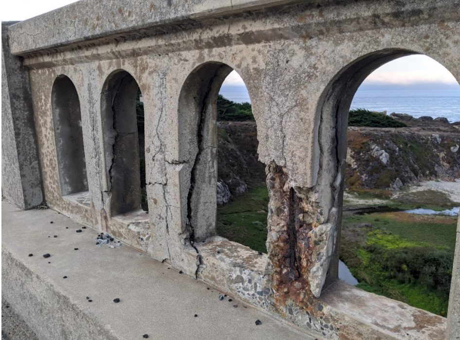
Figure 1-4 Photo of Garrapata Creek Bridge Rail Damage
