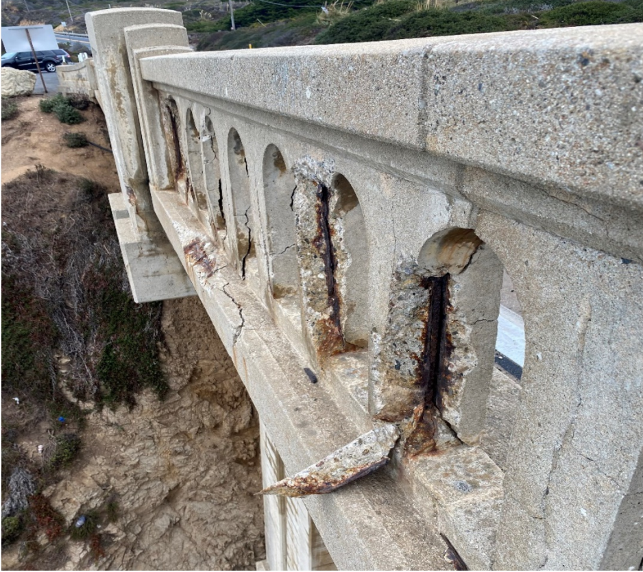
Figure 1-3 Photo of Rocky Creek Bridge Rail Deterioration
