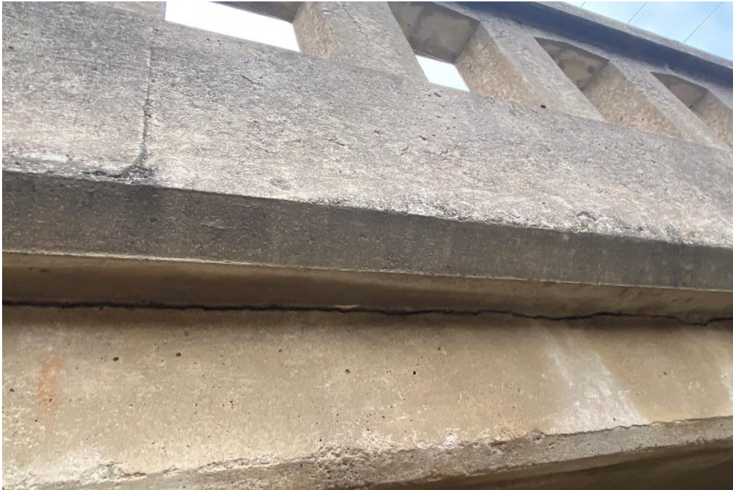
Figure 1-7 Photo of Malpas Creek Bridge Rail Deterioration
