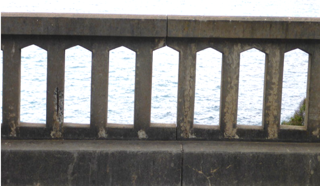
Figure 1-1 Photo of Big Creek Bridge Rail Deterioration
