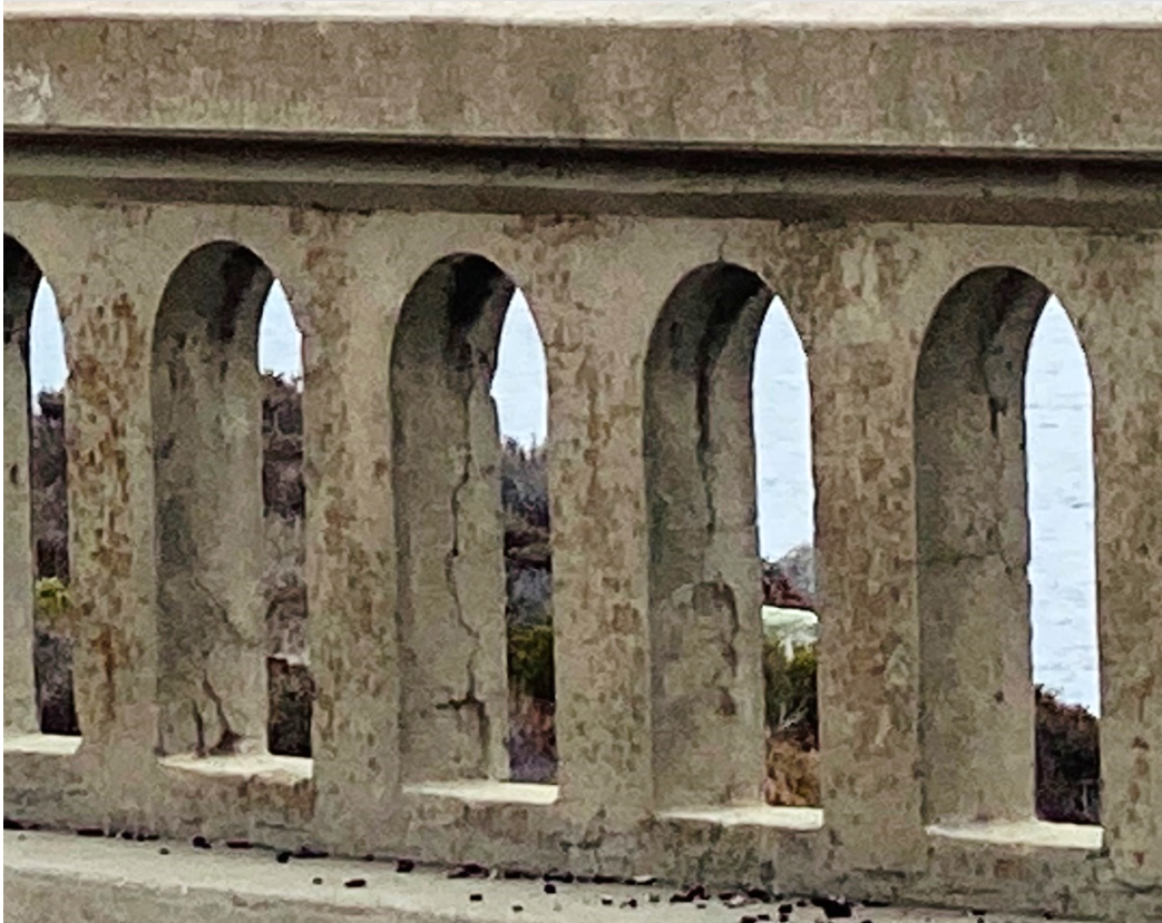
Figure 1-6 Photo of Granite Canyon Bridge Rail Deterioration
