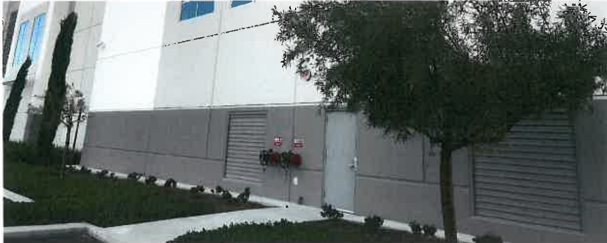
Although provided for illustrative purposes only, the image above shows how ground or wall-mounted equipment would be secured and screened from public viewing areas with landscaping.
