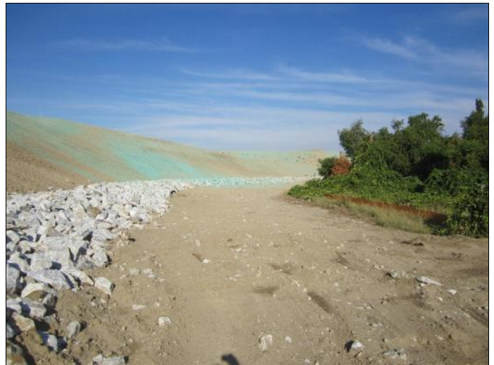
22. View west from southwest corner of subject property and mass grading to the left (south).
