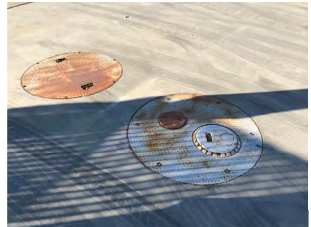
Photograph 6. View of the location of an 1,800-gallon UST in the western portion of the subject property.
