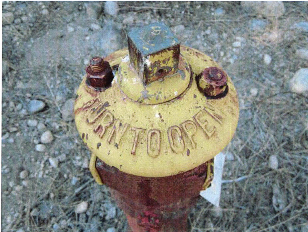
Photo 3. Top of post indicator valve.
