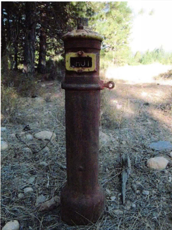
Photo 1. Post indicator valve. Visual indicator showing valve is shut.
