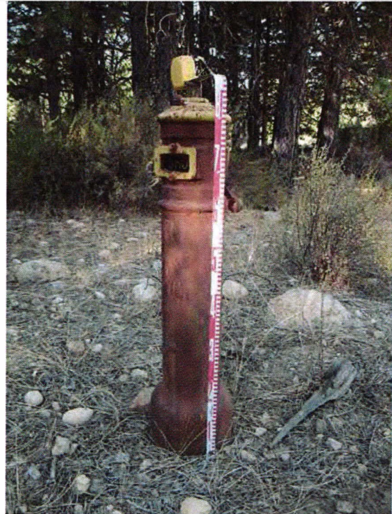
Photo 2. Scale showing height of post indicator valve (87cm / 2' 10")
