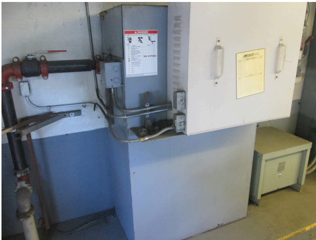
Hydraulic elevator equipment
