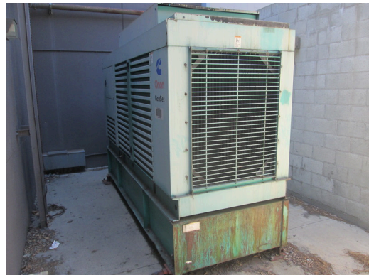
#16 OFFICE BUILDING: EMERGENCY GENERATOR WITH 350-GALLON DIESEL BELLY TANK (AST)
