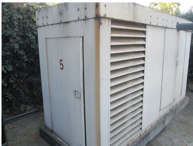
Office Building: Emergency generator with 300-gallon diesel belly tank (AST)
