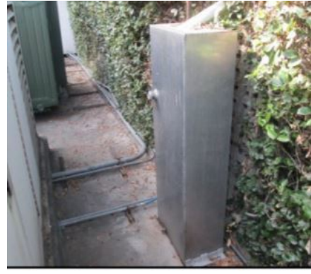
#20 5 GALLON DIESEL AST FOR GENERATOR 1
