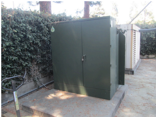
#21 UTILITY-OWED PAD-MOUNTED TRANSFORMER
