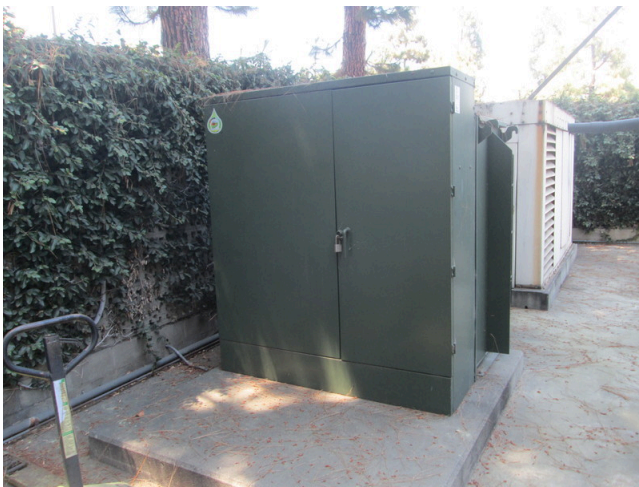
Utility-owned pad-mounted transformer
