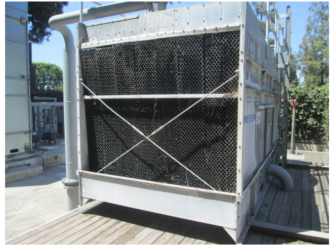
Office Building: Cooling tower
