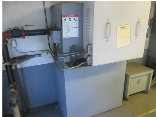
#22 HYDRAULIC ELEVATOR EQUIPMENT
