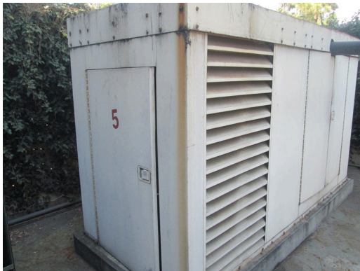
#15 OFFICE BUILDING: EMERGENCY GENERATOR WITH 300-GALLON DIESEL BELLY TANK (AST)
