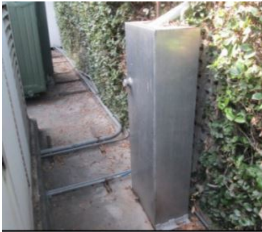
5 gallon diesel AST for generator 1
