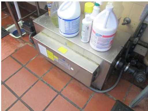
#17 CAFETERIA BUILDING: KITCHEN AREA JANITORIAL SUPPLIES
