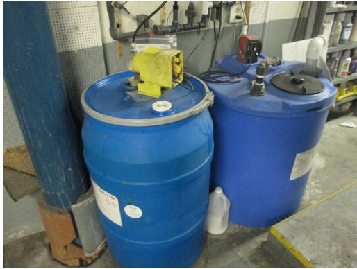
#19 OFFICE BUILDING: HVAC WATER TREATMENT CHEMICALS
