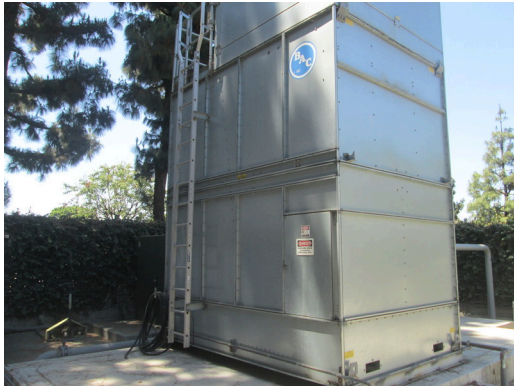
#27 OFFICE BUILDING: COOLING TOWER
