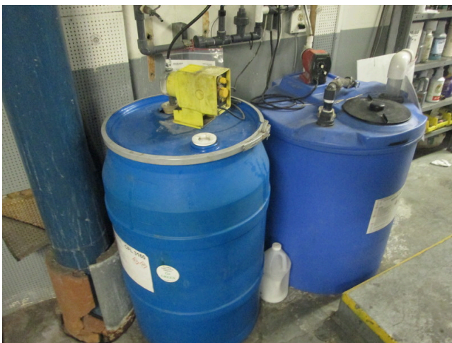
Office Building: HVAC water treatment chemicals
