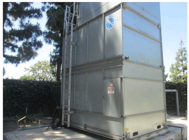
Office Building: Cooling tower
