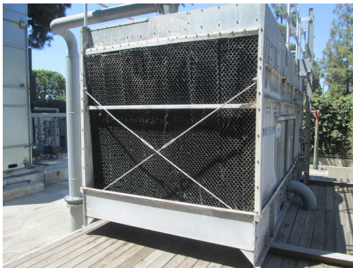
#29 OFFICE BUILDING: COOLING TOWER
