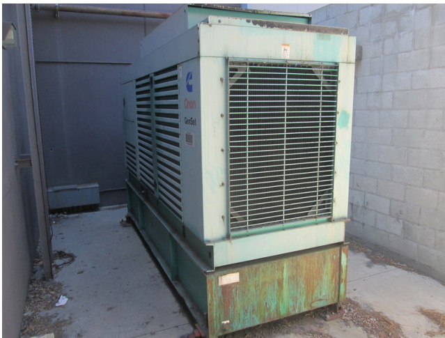
Office Building: Emergency generator with 350-gallon diesel belly tank (AST)
