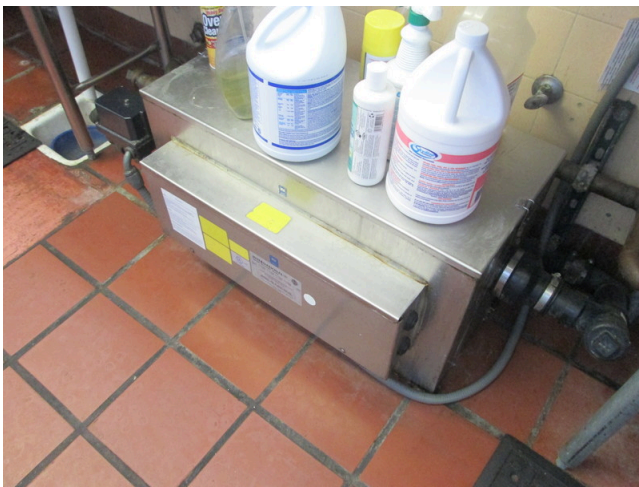
Cafeteria Building: Kitchen area Janitorial supplies
