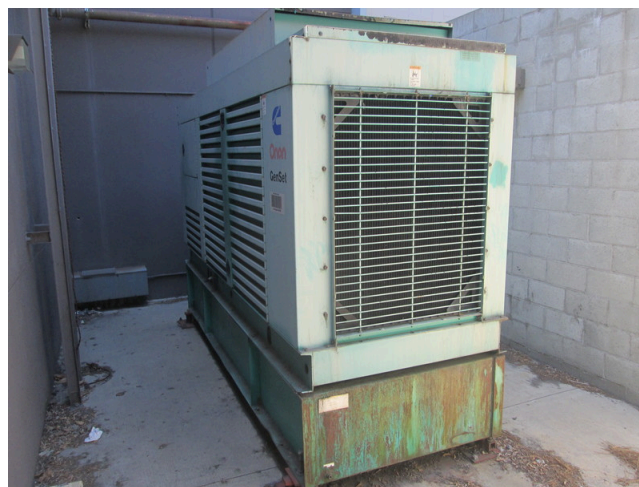
Office Building: Emergency generator with 350-gallon diesel belly tank (AST)
