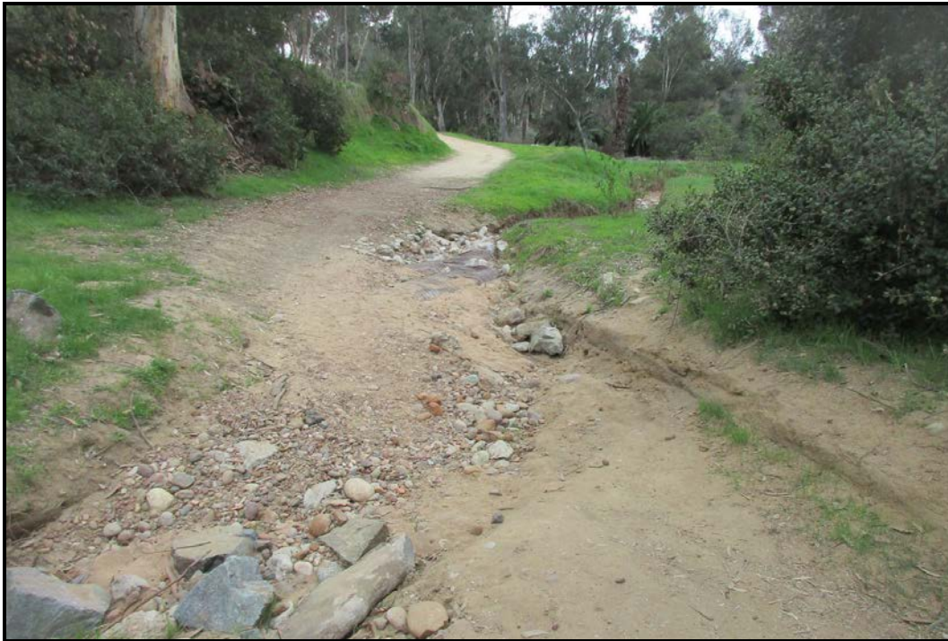
PHOTOGRAPH 1 Main Storm Drain along Trail with Some Erosional Cuts, Looking Southwest
