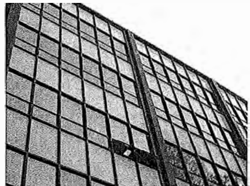
North face of six-story annex curtain wall. Note open windows on the fourth floor.
