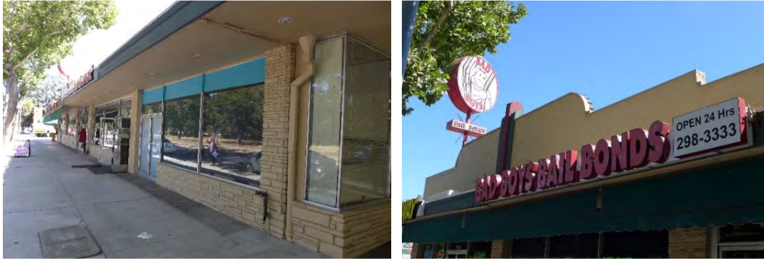
Figures 33 and 34. The 1086-1096 N. First Street storefronts (left) and the parapet detail (right).
