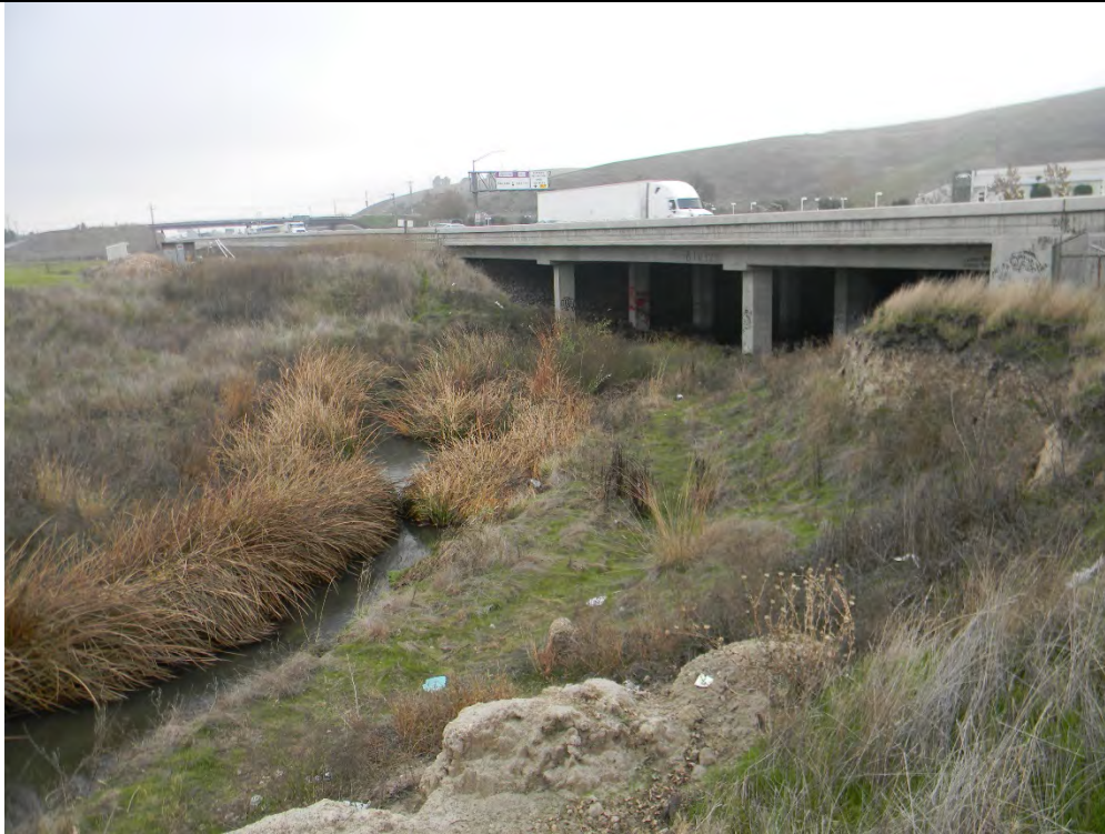
6. Photograph from the northwest of Arroyo Las Positas flowing underneath Arthur H Breed, Jr Freeway
