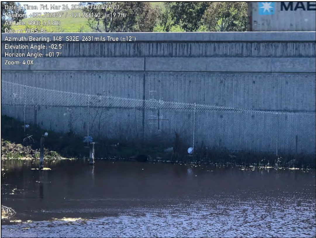
Looking south at I-580 and culvert entrance that connects Feature 6 to Arroyo Las Positas.
