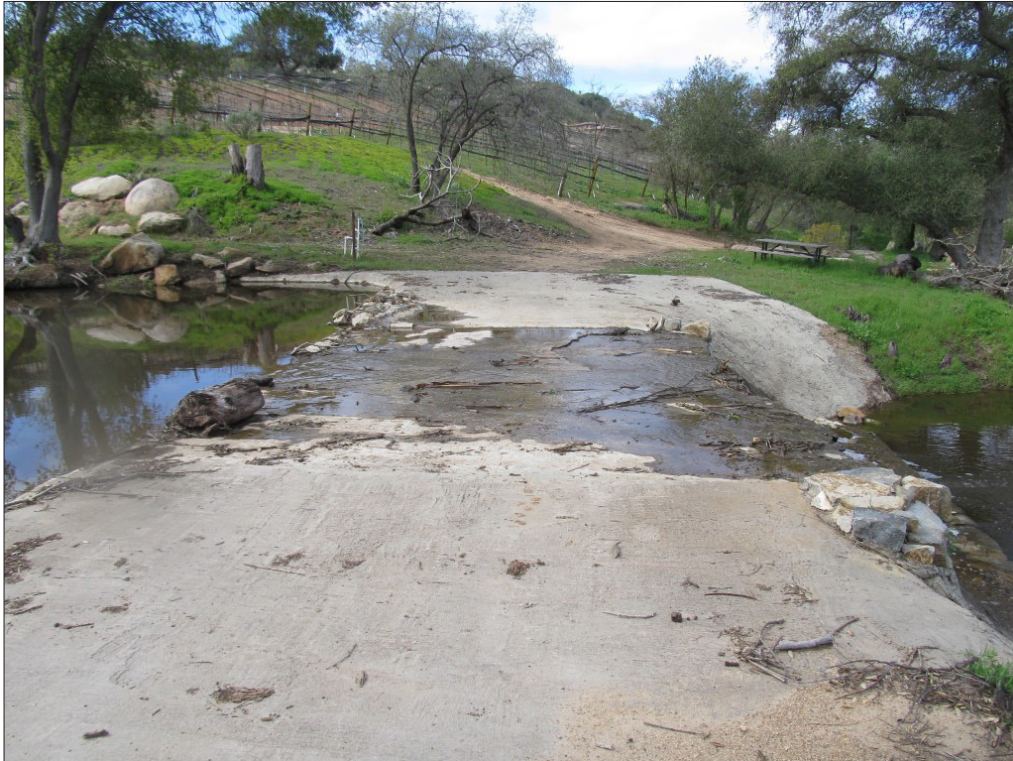
Photo 11. View of the concrete Arizona crossing/spillway that separates the second and third manmade seasonal ponds, looking west. Photo taken February 28, 2019.
