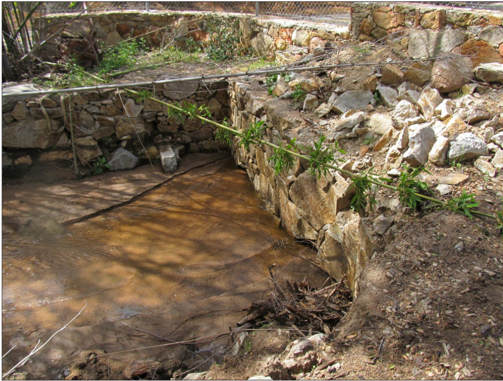
Photo 6. View of the same roadside ditch shown in Photo 5, looking southwest. Photo was taken after subsequent rain events and shows flowing water and substantial sediment deposition above the sediment-clogged culverts. This feature was mapped as potential jurisdictional waters. Photo taken February 28, 2019.
