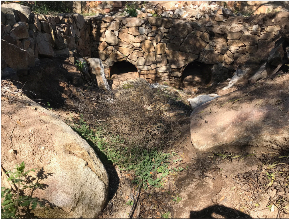
Photo 5. View of a roadside ditch at the southeastern corner of the site, looking northwest toward two culverts full of sediment underneath the eastern driveway. Photo shows no ponded or flowing water or evidence of water flow or ponding, despite recent rains. Photo taken February 8, 2019.
