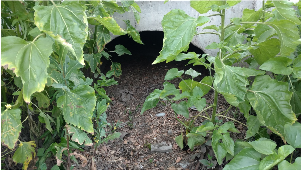
Photograph 3 – Ditch 1 starting point. Culvert west of Ashwood Street and north of Mapleview Street, facing east.
