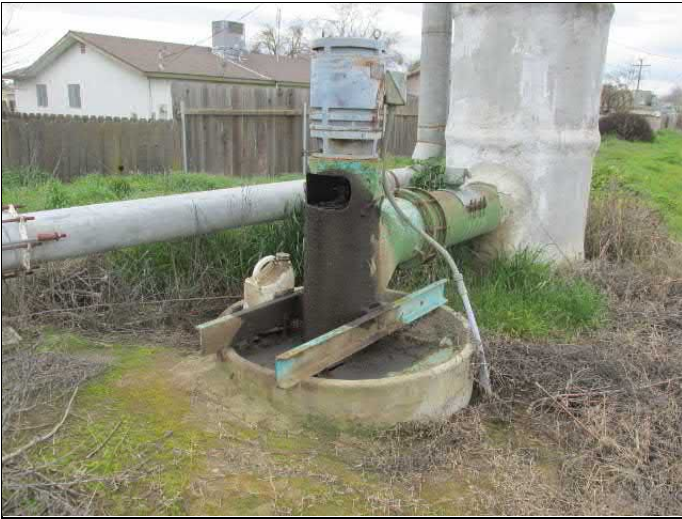
19. View of a lift pump within the southern portion of the subject property.
