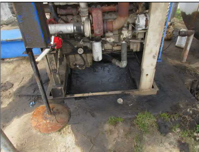
17. View of the lubrication oil surface staining beneath the engine.
