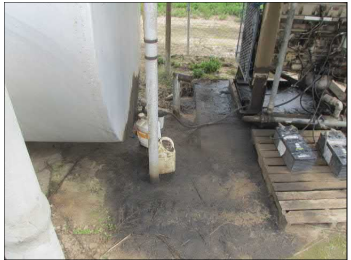
16. View of the lubrication oil surface staining between the diesel AST and associated engine.
