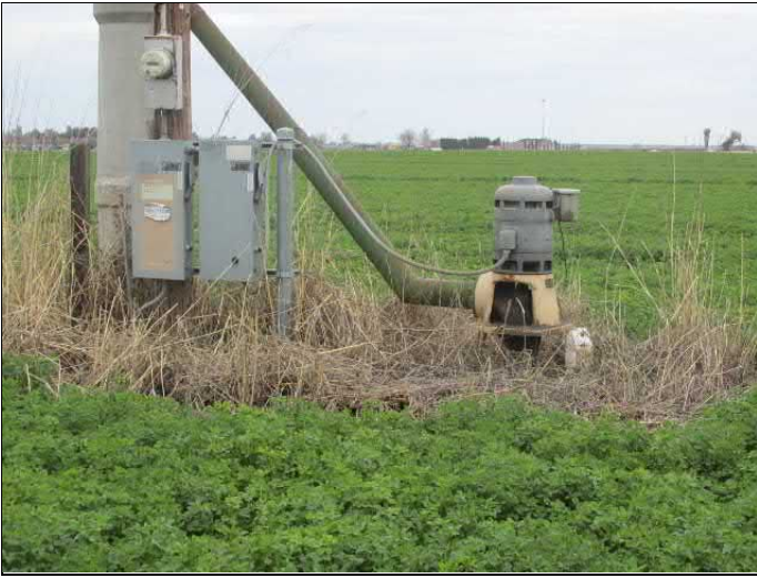
13. View of an electrically powered irrigation well.
