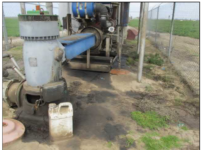
18. View of the diesel-powered irrigation well and de minimis lubrication oil surface staining.
