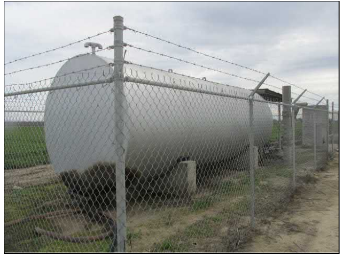
14. View of a 10,000-gallon diesel AST located within the central portion of the subject property.
