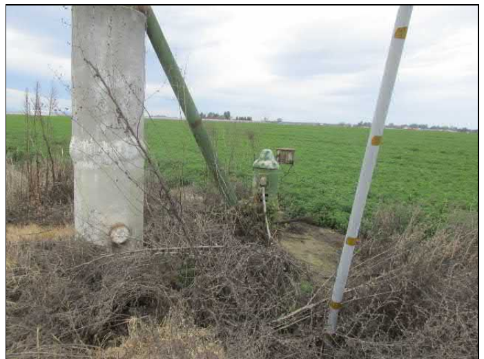
12. View of an electrically powered irrigation well.
