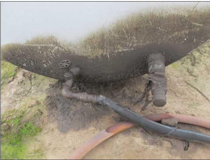
15. View of de minimis diesel surface staining beneath diesel AST valve.
