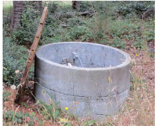
Well #2 Concrete Caisson Enclosure with Wood Lid
