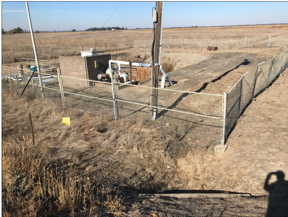
Photograph 3: Storm Water Treatment, looking south from County Road 28H.
