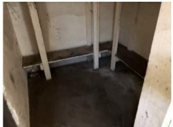
Photo #72 View of the container room in the milk barn after cleanup and removal. Refer to Photos #14 and #15.
