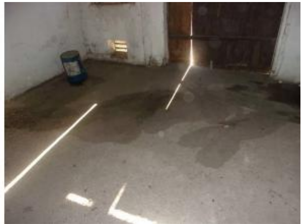
Photo #16 Additional view of concrete staining extending from the room located on the southern portion of the milk barn as seen in Photos #14 and #15.
