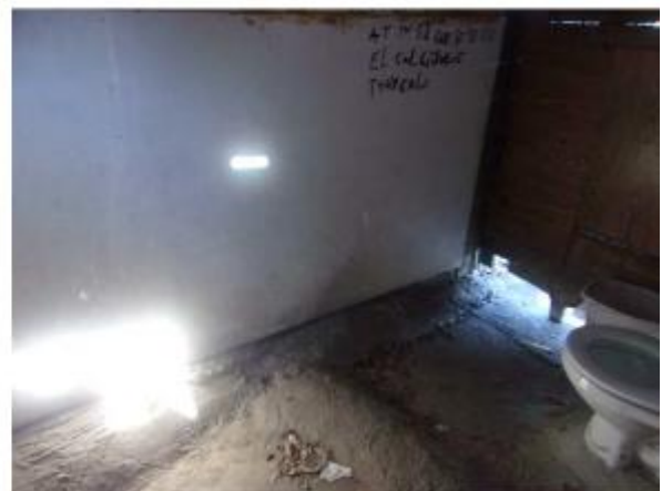
Photo #36 View of restroom and floor drain inside the building seen in Photo #35 (arrow).
