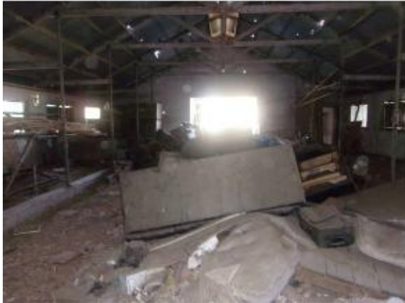
Photo #13 View of household trash and debris piles located on the northern portion of the milk barn.
