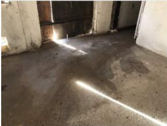
Photo #73 View of the staining in the milk barn after cleanup. Refer to Photo #16.
