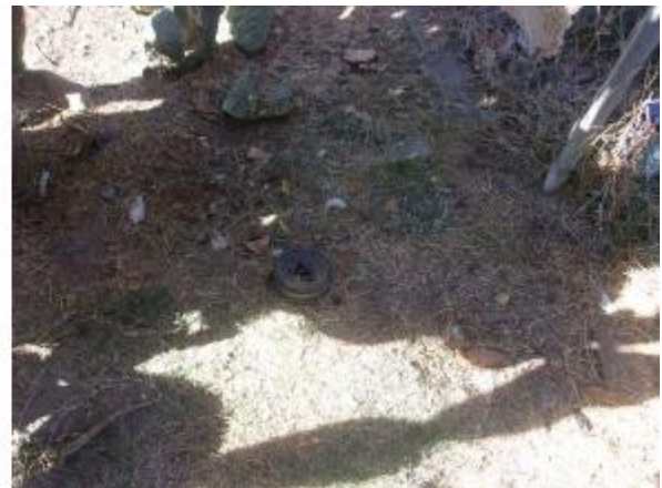
Photo #12 View of the septic system clean out located on the west side of the occupied residence (6735 W. Grant Line Road).
