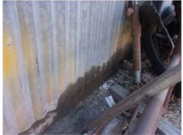
Photo #26 View of staining along the northern edge of the shop/garage building exterior wall opposite the air compressor seen in Photo #25.
