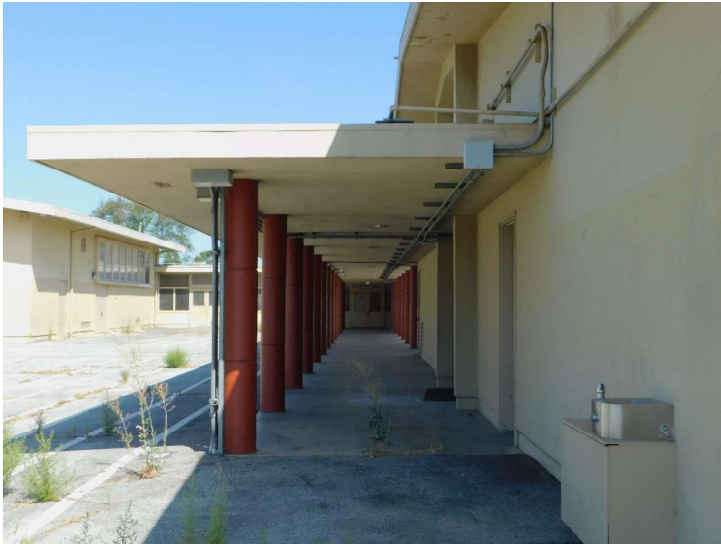
Figure 14. Covered Walkway connecting Buildings A and B, looking N towards Building A (DSCN3790)
