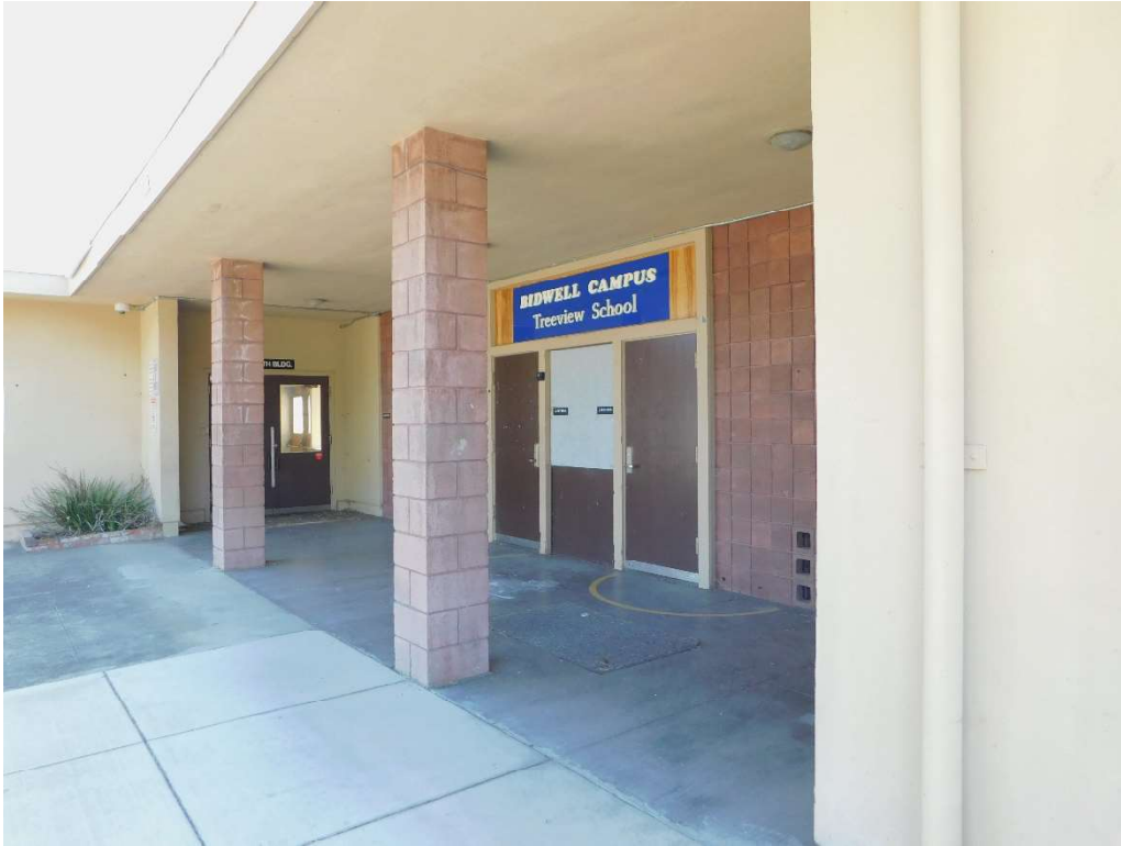
Figure 4. Recessed entry on the north (main) elevation showing sienna CMU details, looking SE (DSCN3750)
