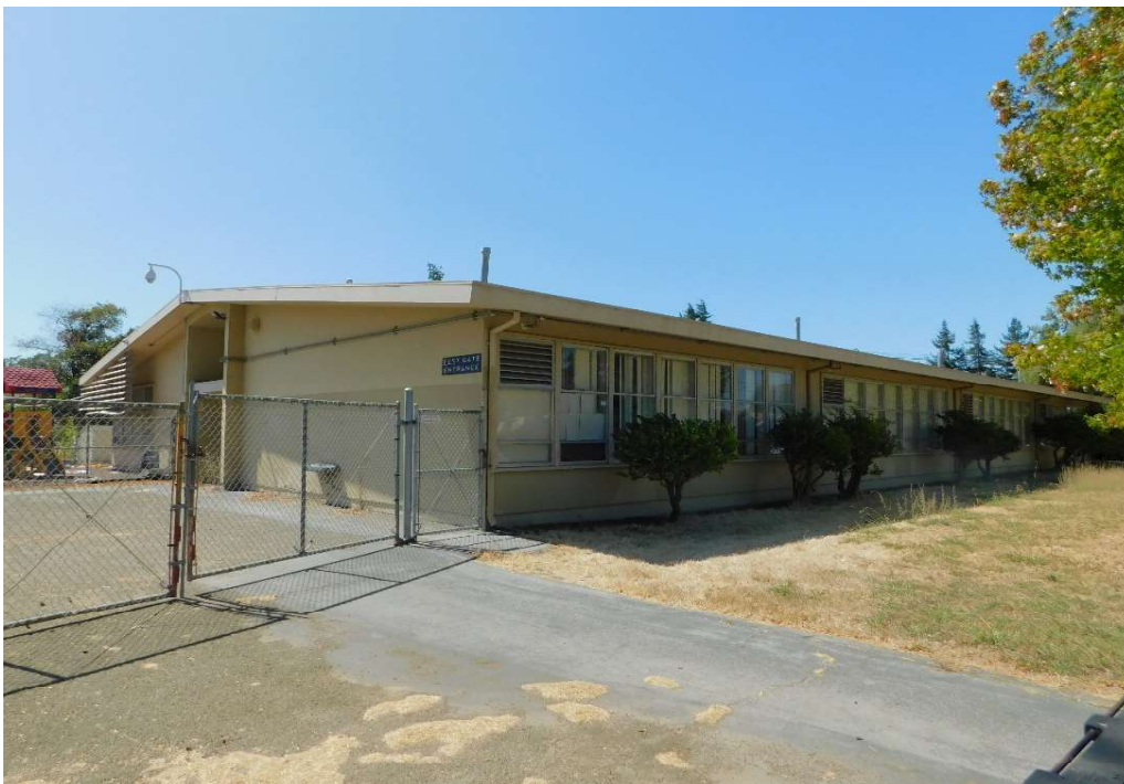
Figure 7. North (main) and east elevation showing protruding framed entry, looking SW (DSCN3853)
