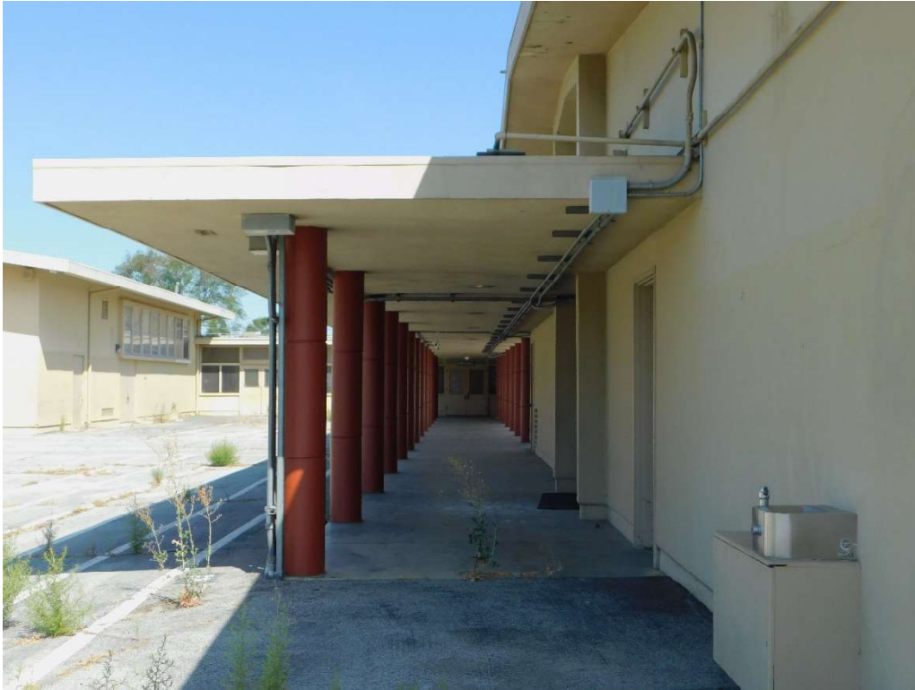
Figure 8. Covered Walkway connecting Buildings A and B, looking N towards Building A (DSCN3790)
