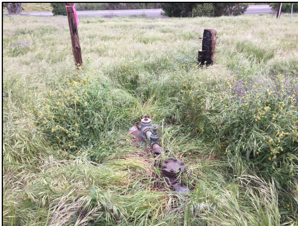
Plate 4.6–1: Overview of the remaining pipes and valves at Site P-33-015672, facing north.
