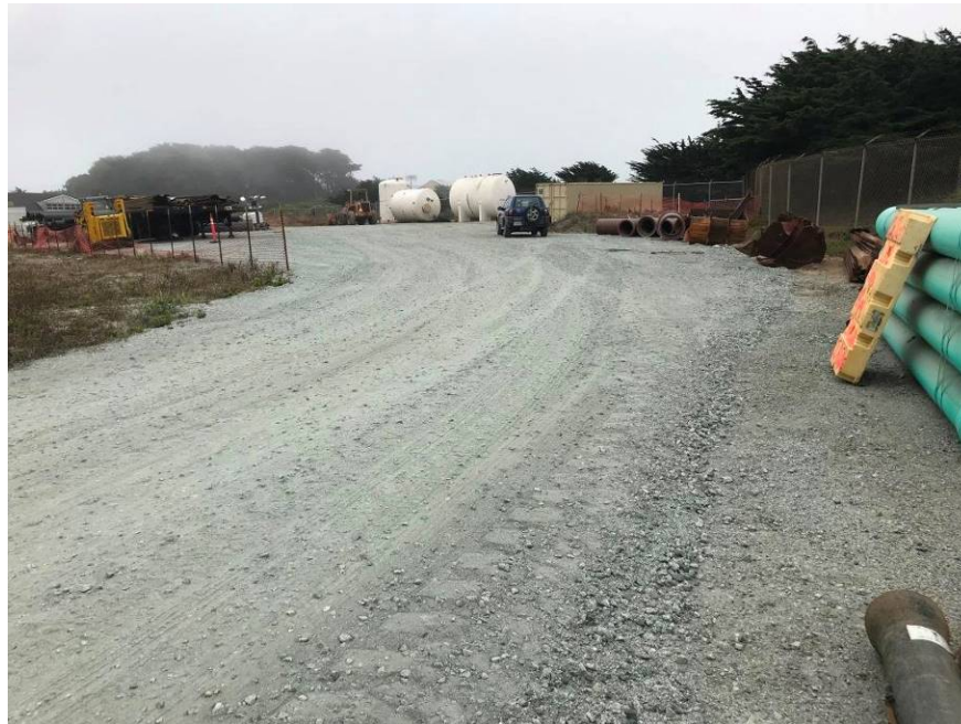
Photo 6: Staging area 4 is all aggregate base. It is an active staging area with no vegetation establishment, except for ruderal plants on the edge. Photo taken on July 16, 2019, looking southeast from the access road to this area.
