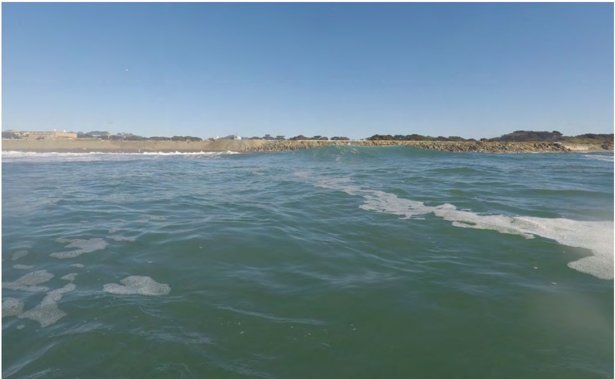
Photo 12. Offshore view of north end of revetment near Westside Pump Station, facing east
