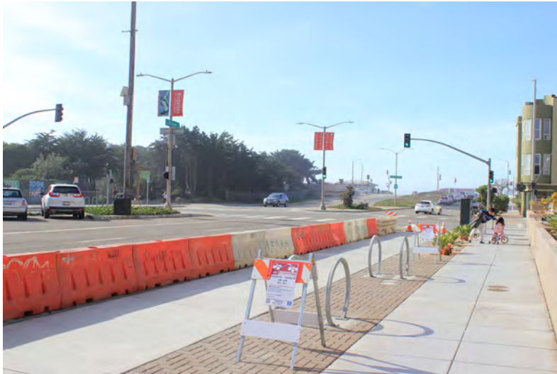
Photo 5. View towards the Sloat Boulevard zoo entrance and the Great Highway, facing west.
