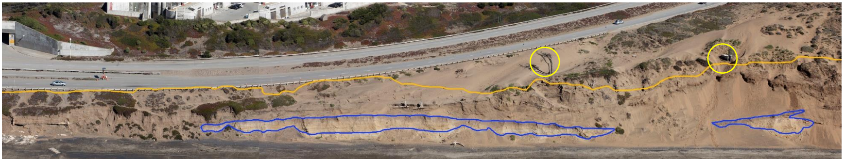
CCR imagery from October 1, 2009 shows substantial coastal erosion since 2004 and a related reduction in bank swallow habitat. The approximate 2019 bluff line is shown in orange.
