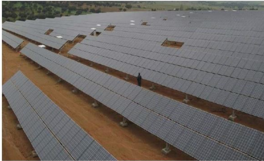
Typical Fixed-Tilt Solar Panel Rows
