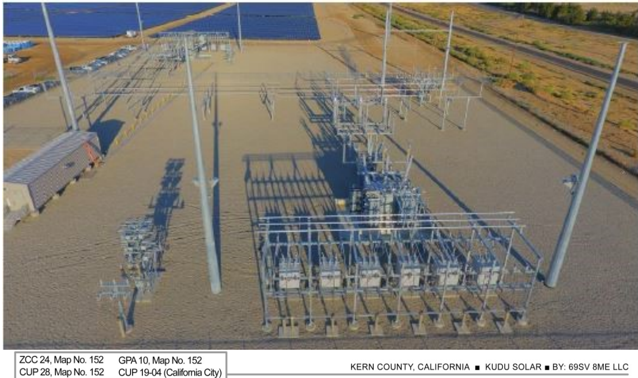
Figure 3-19. Representative Example of Typical Substation Design
