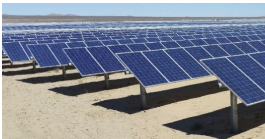
Typical Single-Axis Tracking Solar Panels
