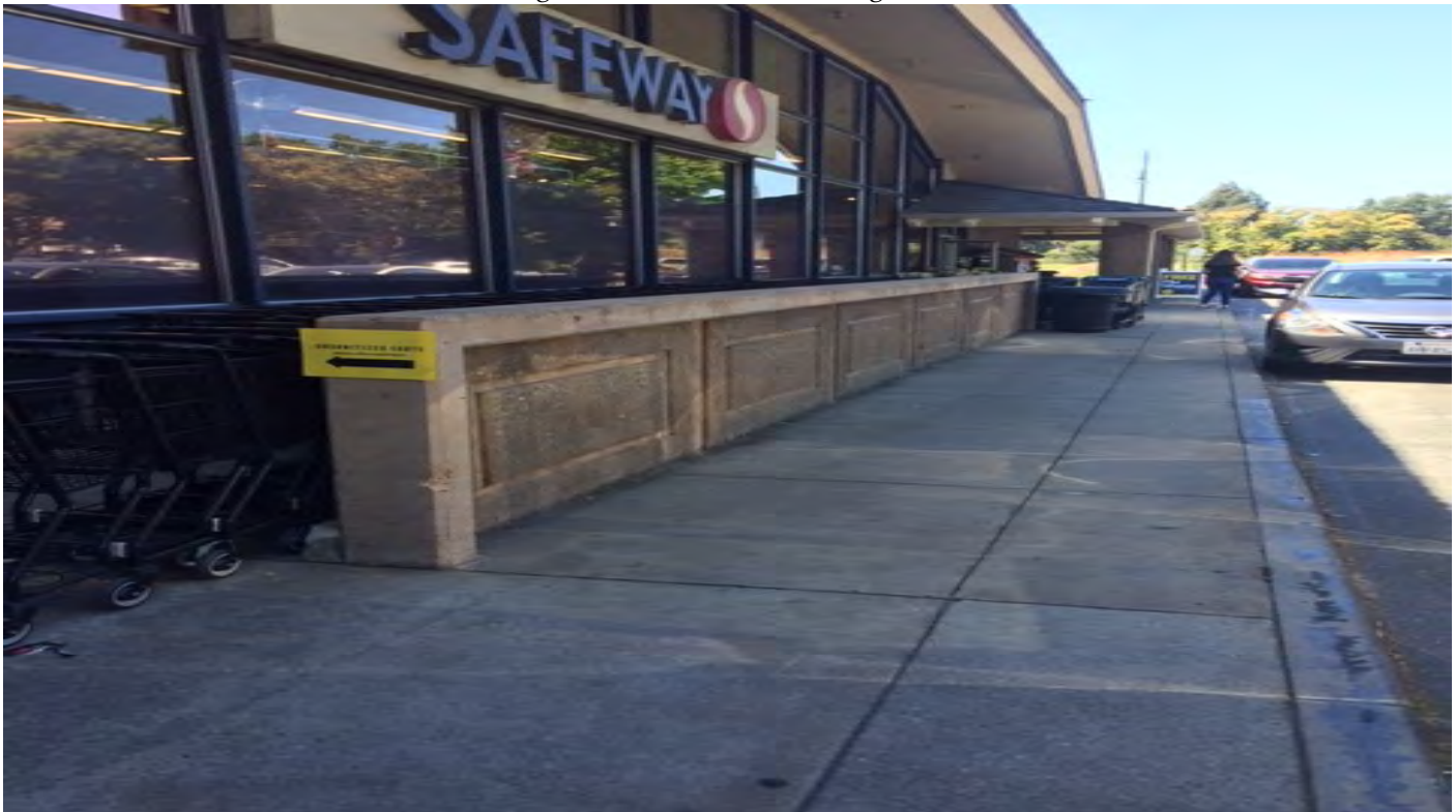
Figure 5. Concrete wall obscuring front elevation
