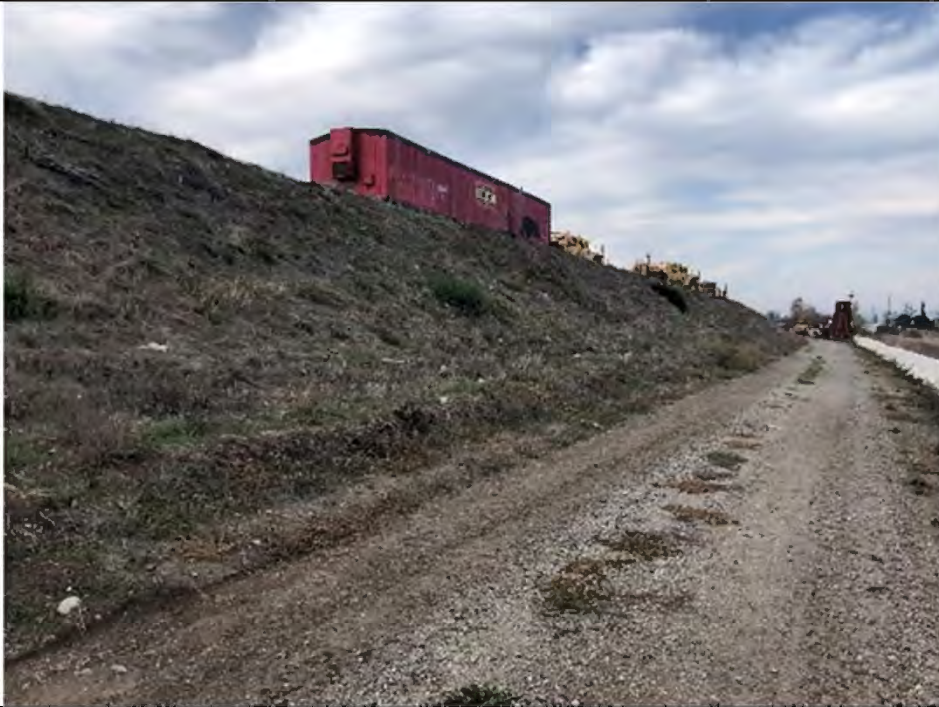
Concrete k-rail (right) prevents CTS from accessing (dispersing onto) the site. Berms are comprised of fill material and do not provide suitable estivation habitat for CTS.
