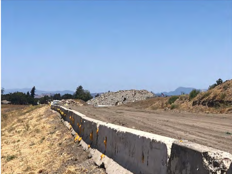
Concrete k-rail is maintained regularly and backfilled on the interior to prevent CTS from dispersing onto site. K-rail also acts a barrier to prevent accidental discharge to adjacent wetlands and drainage ditches (shown on left).
