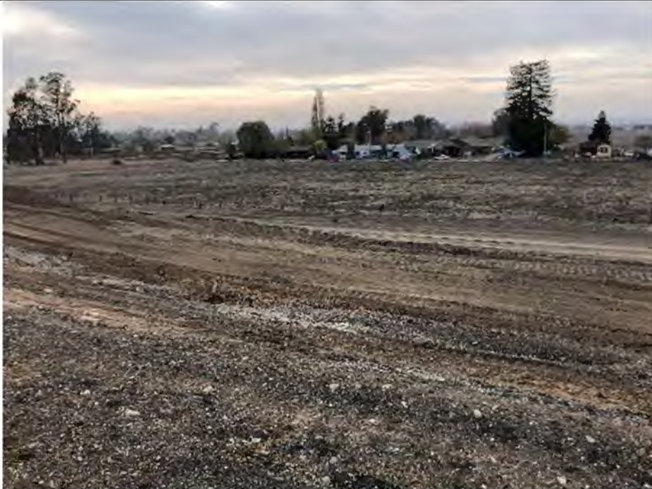
West facing photo taken from top of berm looking out onto dirt roads and adjacent disked agricultural parcel; site compaction and fill precludes CTS.
