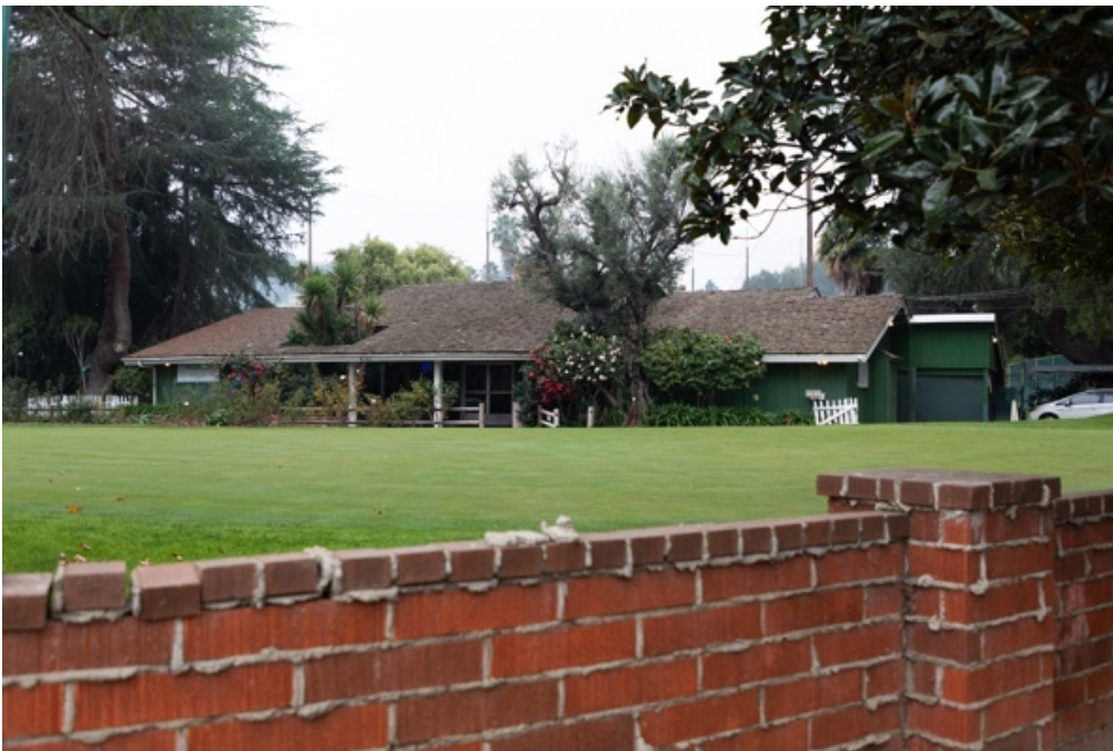
Photo 4. Clubhouse, putting green, and low brick wall with weeping mortar, view facing southwest.
