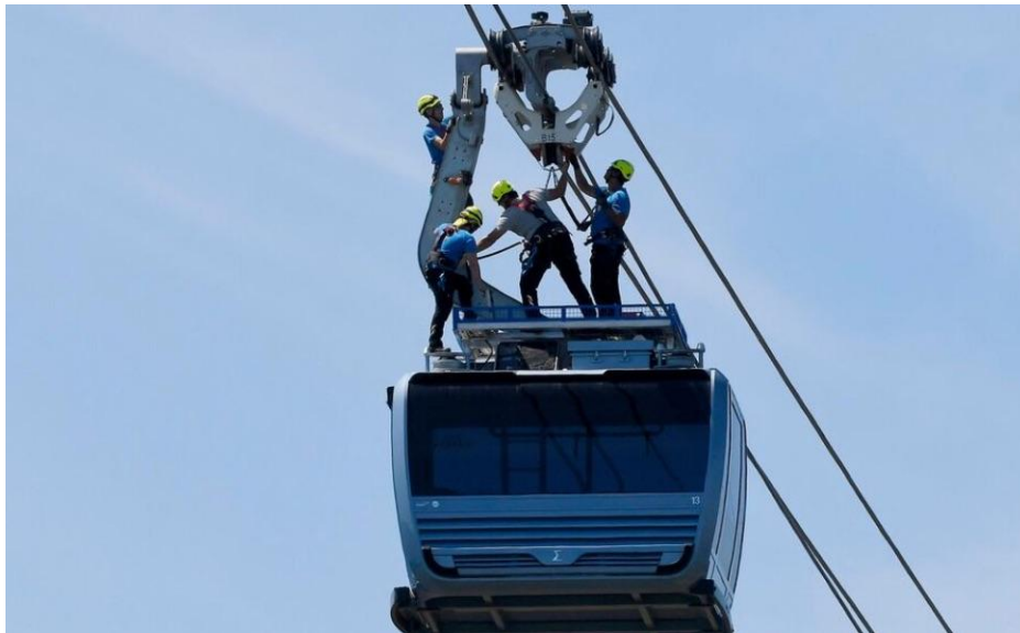
Workers performing repairs on Toulouse 3S Teleo Gondola, which suffered several breakdowns during the first month of service.
