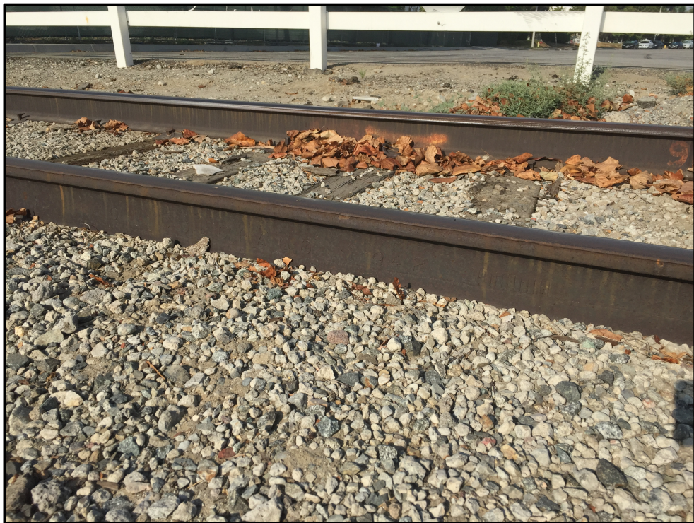
Plate 4.2-8: Close-up view of the rails found within the off-site improvement area, facing west.
