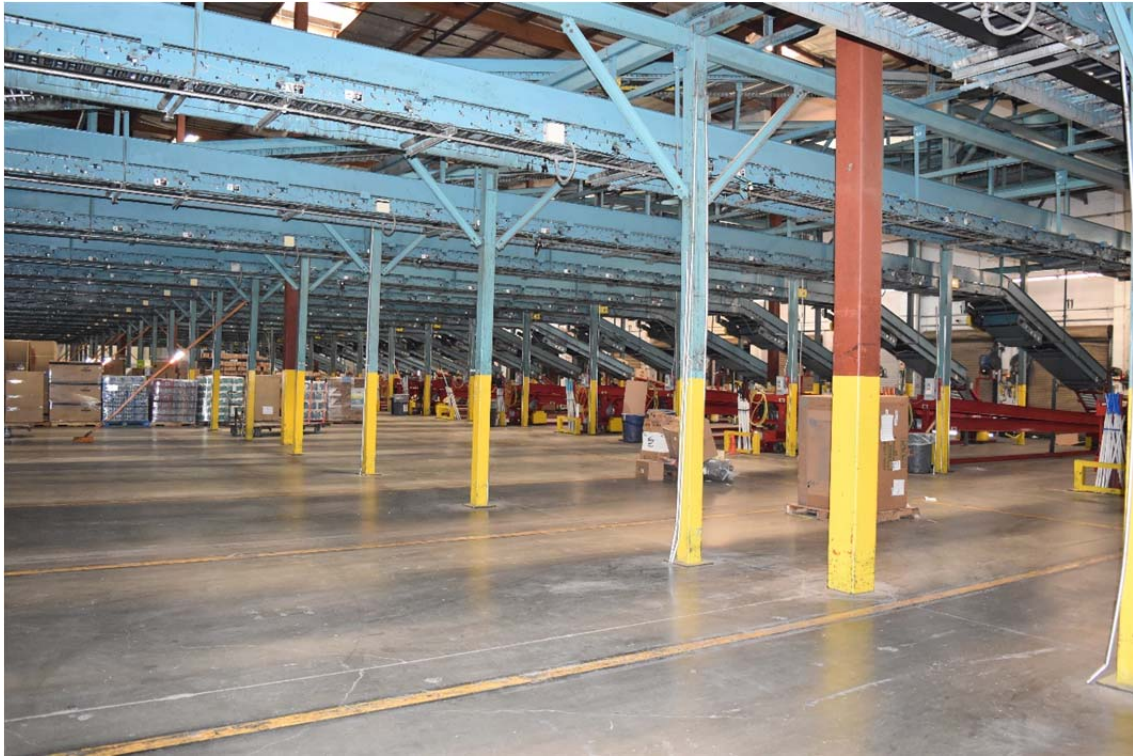
35. Conveyor belts for transporting received goods throughout the structure.
