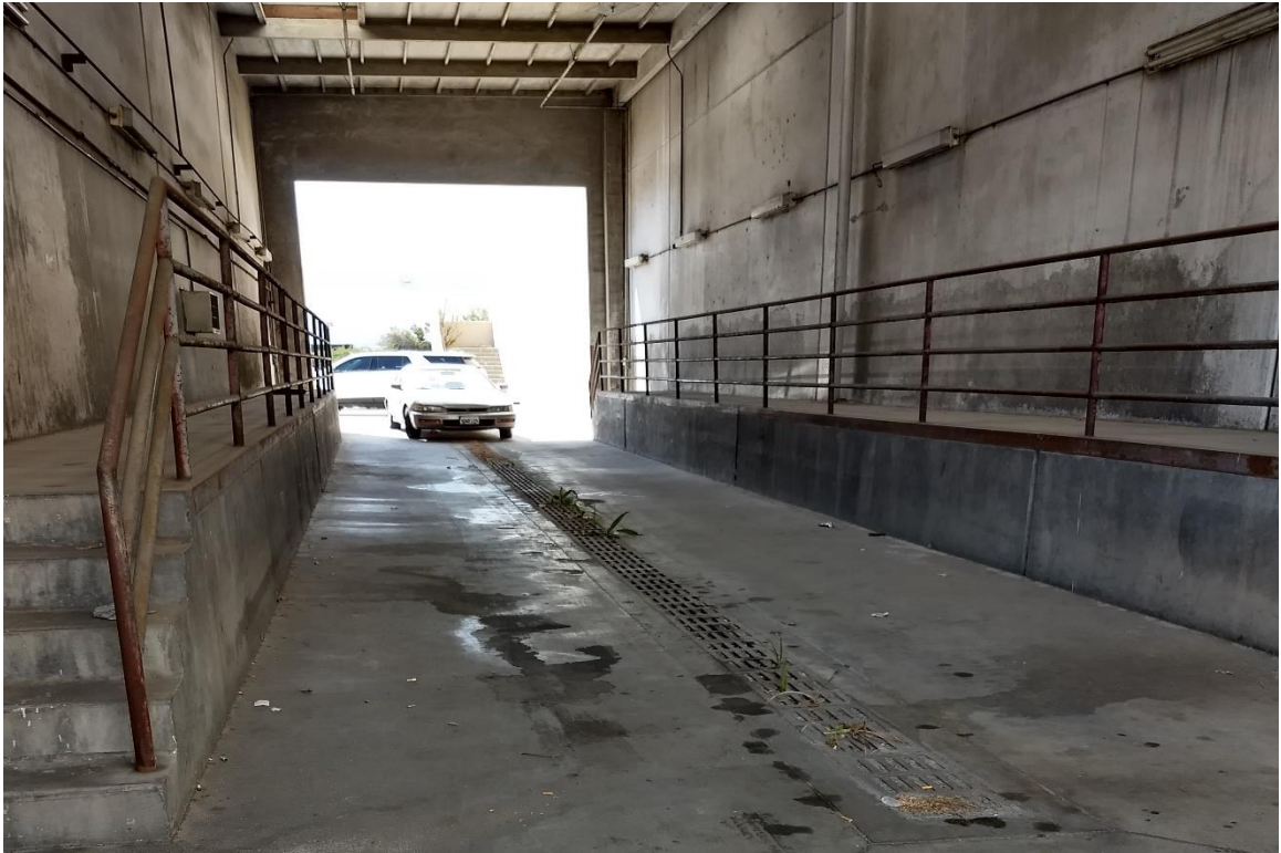
Photograph No. 3: Former Truck Wash located on the northern portion of the Former Truck Maintenance Area.
