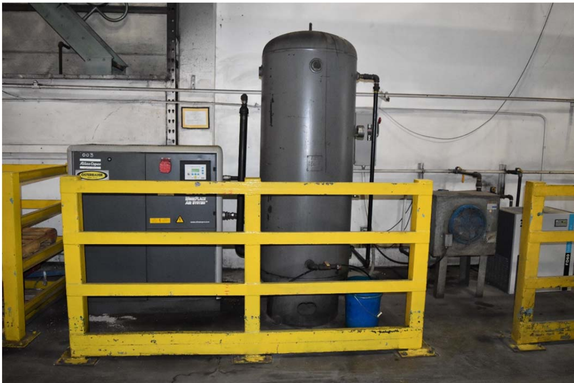
38. Compressor used to power the conveyor belt system in the southeastern portion of the structure.
