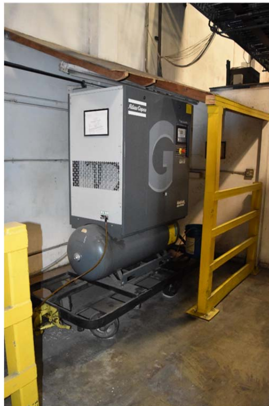
36. Compressor used to power the conveyor belt system in the southeastern portion of the structure.
