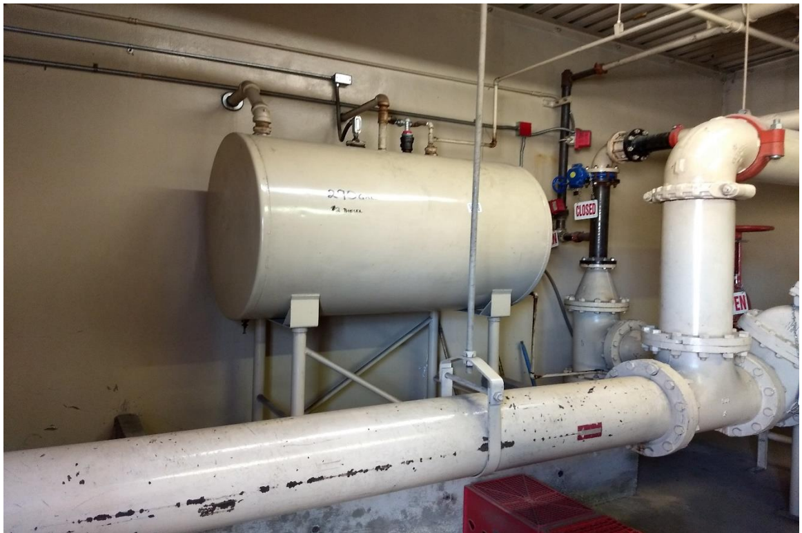
Photograph No. 10: Pump House diesel fuel aboveground storage tank (AST).
