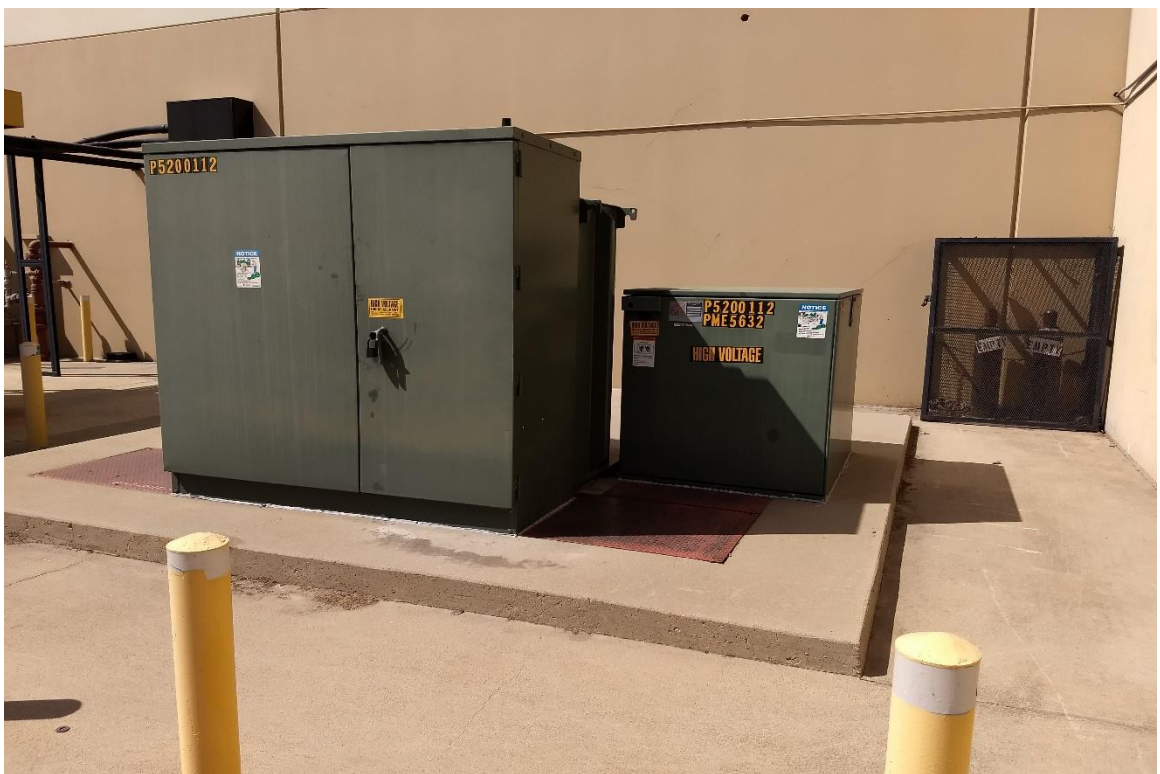
Photograph No. 8: Two pad-mounted electrical transformers immediately south of the Warehouse Building, looking north.
