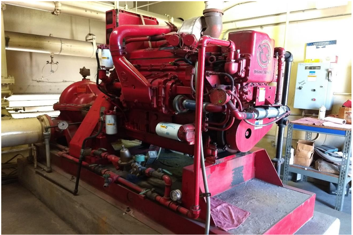
Photograph No. 11: Pump House pump and internal combustion motor.
