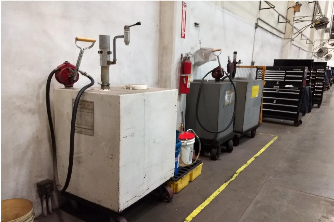
Photograph No. 15: Mobile oil ASTs in the Forklift Maintenance Area.
