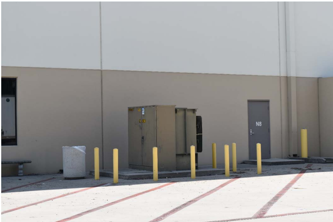
14. Transformer located outside of the northern portion of the warehouse structure.
