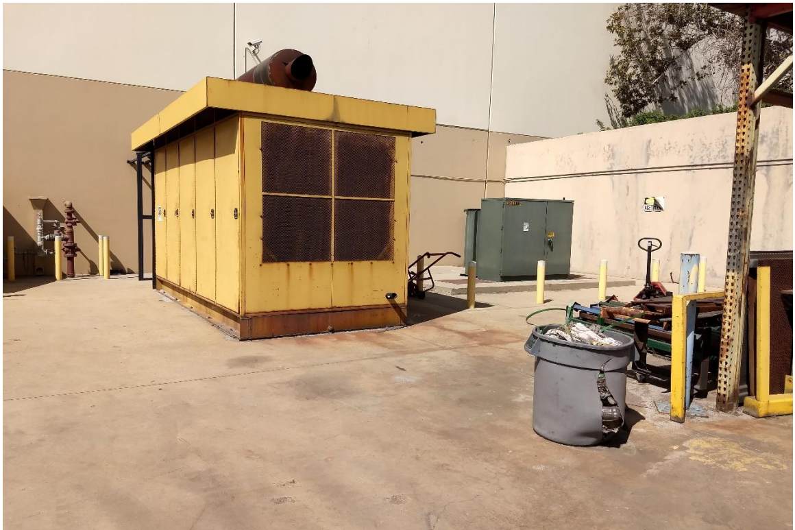
Photograph No. 7: Emergency generator located immediately south of the Warehouse Building, looking north.
