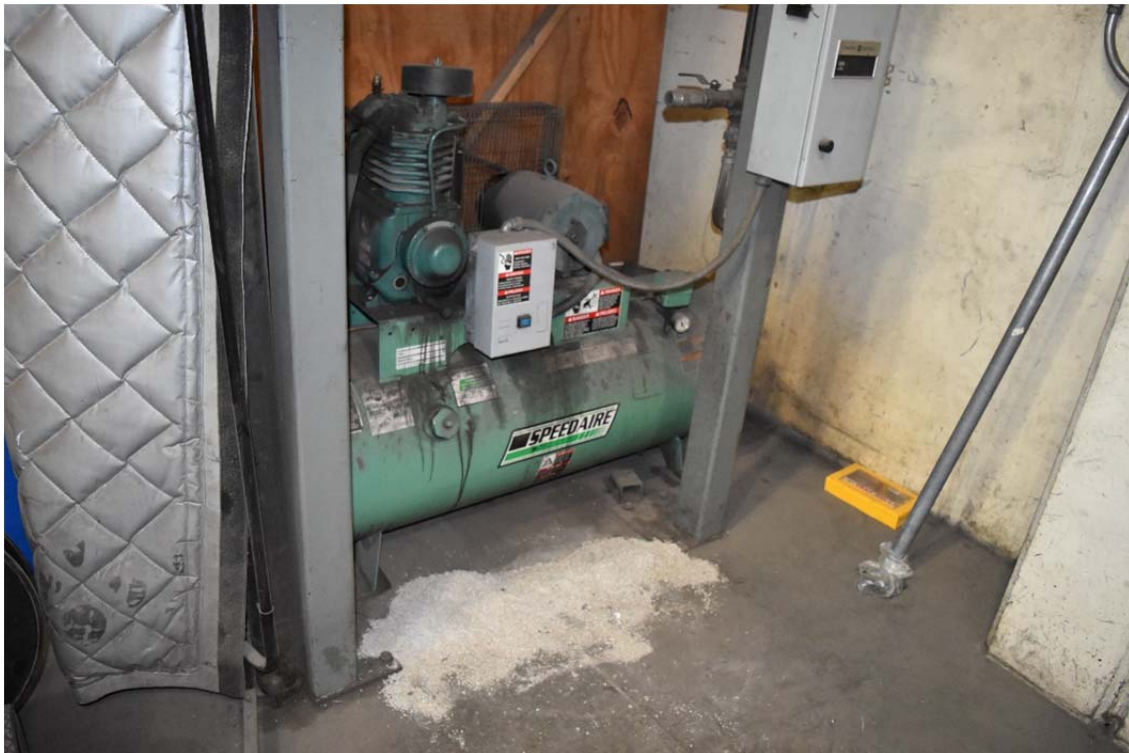
28. Compressor located in the maintenance area in the southern portion of the structure.
