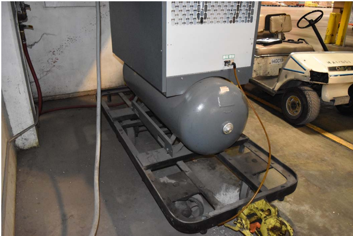
37. Compressor used to power the conveyor belt system in the southeastern portion of the structure.
