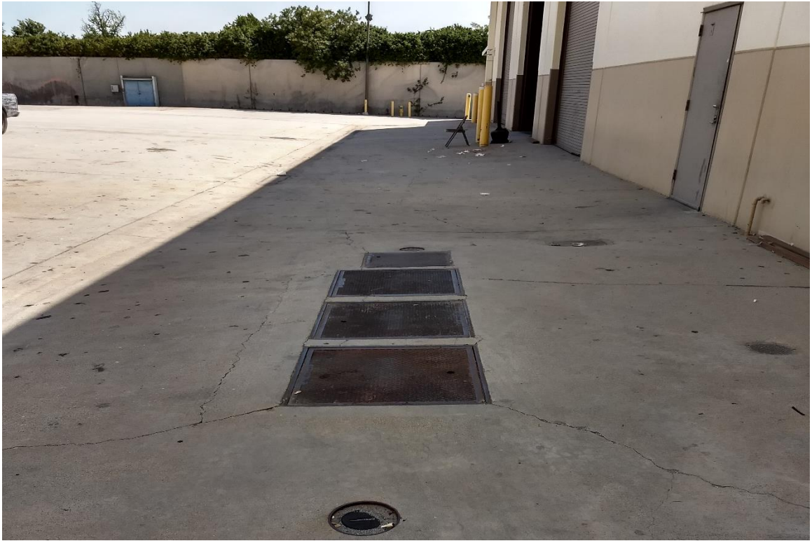
Photograph No. 5: Clarifier located immediately east of the Former Truck Maintenance Area, looking south.
