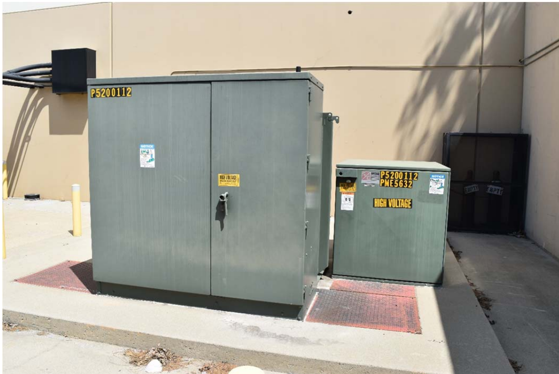
51. Transformer located to the east of the former automobile maintenance area and south of the warehouse structure.
