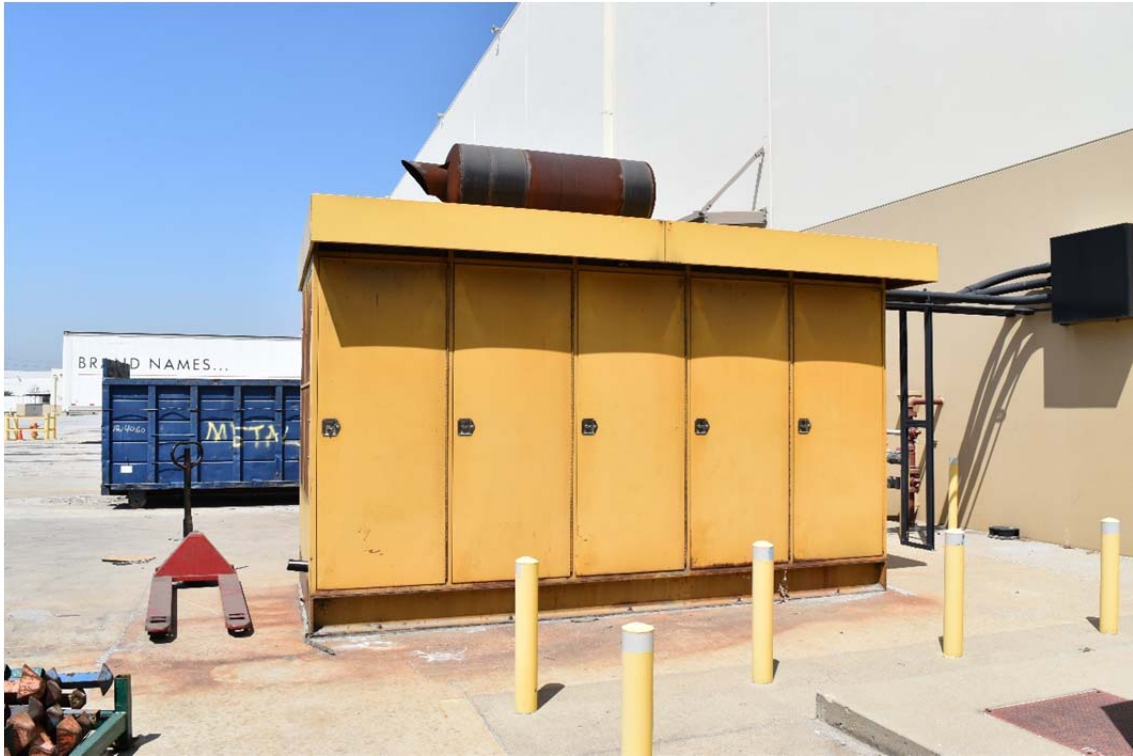
49. Diesel powered emergency back-up generator located to the east of the former automobile maintenance area and south of the warehouse structure.
