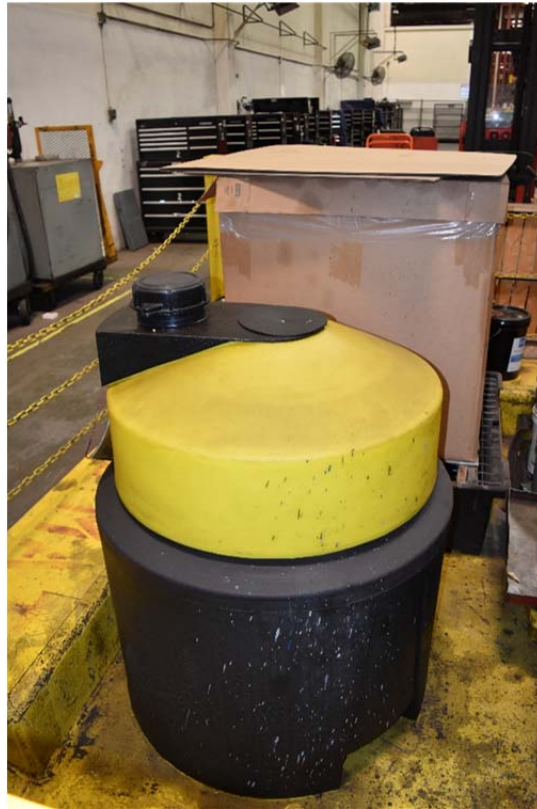
27. Waste oil storage drum within secondary containment in the maintenance area of the structure that are routinely removed under proper manifest.
