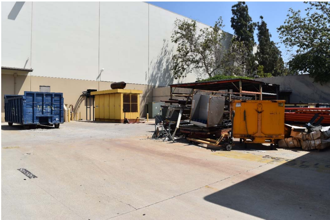
48. Emergency back-up generator (diesel-powered), dumpster, transformer, and material storage area outside to the east of the former automobile maintenance area.
