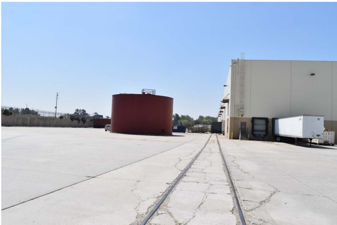
16. Aboveground tank for the storage of water for emergency fire suppression services with small adjacent structure for emergency generator on the eastern portion of the Site – view facing south.
